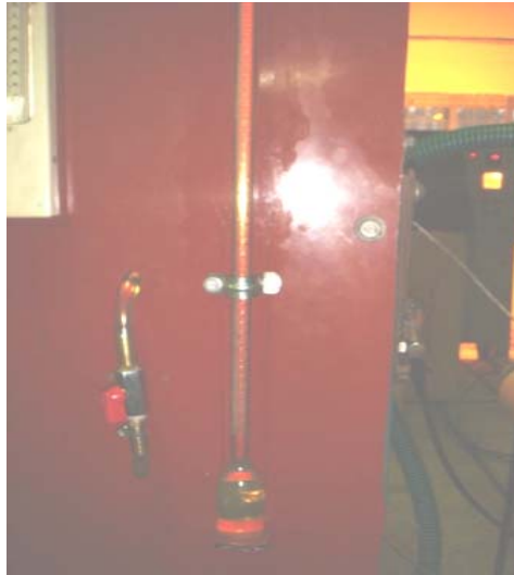
Plate 3.5: Fuel Consumption Measuring Unit
