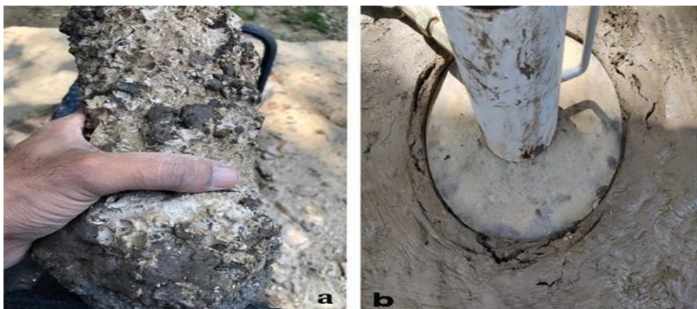
Figure 4.17 (a) Bulb is developed at the base of the column due to punching failure; (b) cracks developed at the surface due to punching
