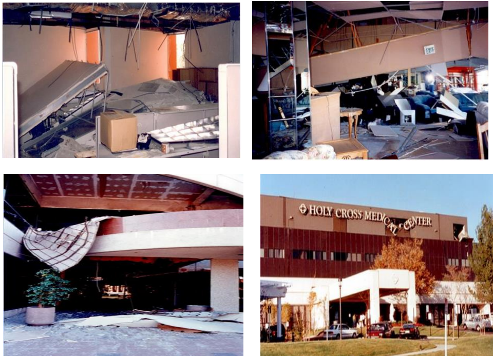
Figure 1.2 Failure of office partitions, ceilings, light fixtures, heavy soffit and HVAC.[9]
