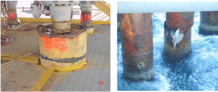
Fig. 1.5. Cracked Tubular Joints. Ref: https://madcon.com/
