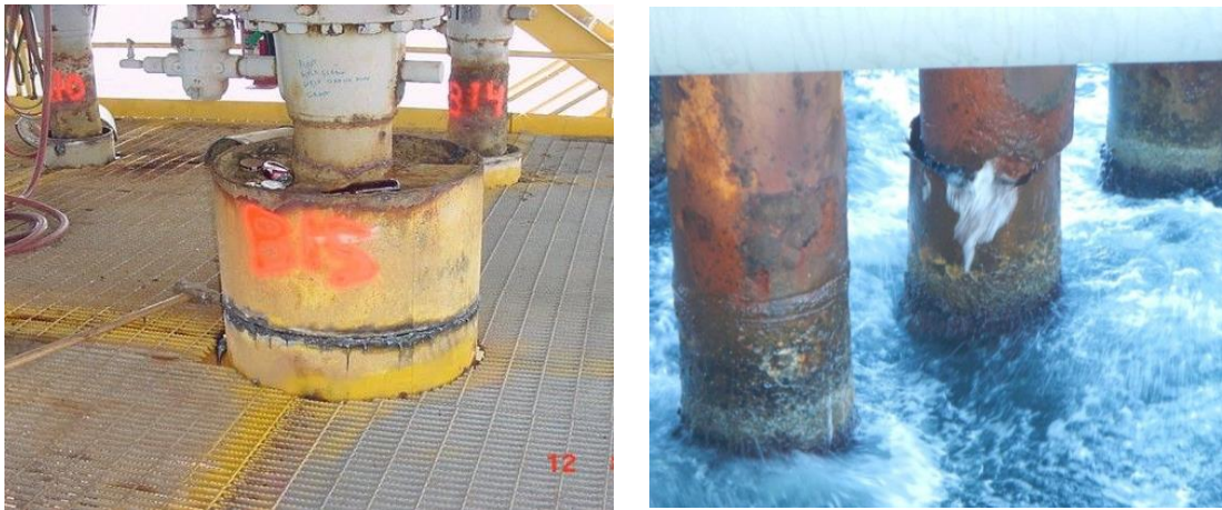
Fig. 1.5. Cracked Tubular Joints
