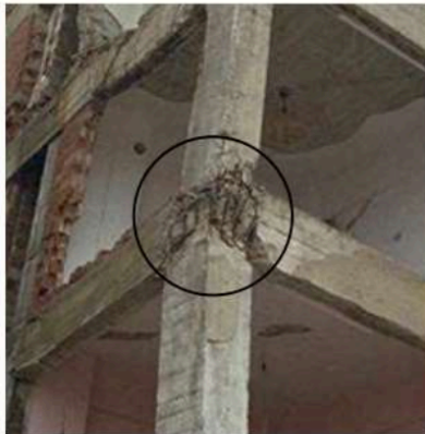
(b) Close-up of beam-column joint failure
