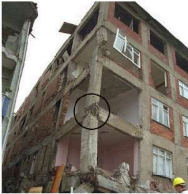
(a) Failure of beam-column joint
