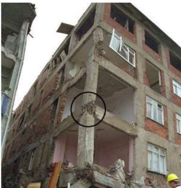
(a) Failure of beam-column joint
