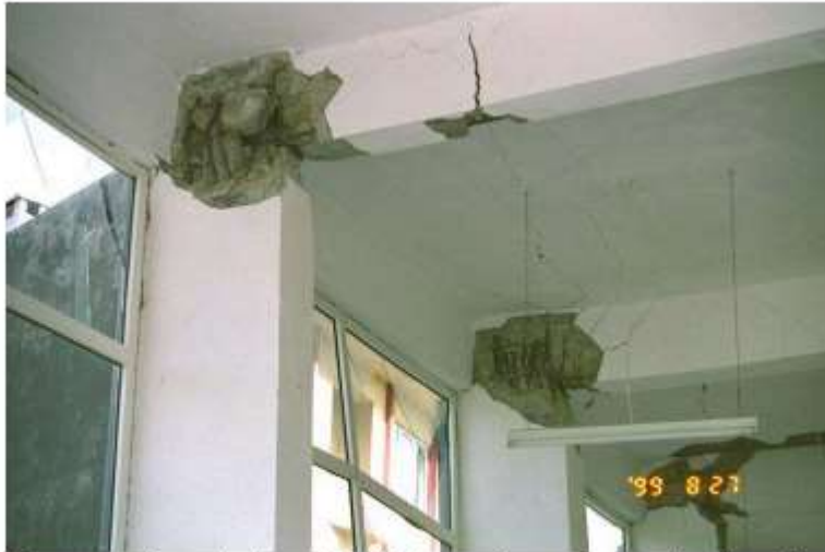
(c) Damage to beam-column joint of building under construction in Adapazari, Turkey (Image source: http://nisee.berkeley.edu/elibrary/Image/IZT-749 )
