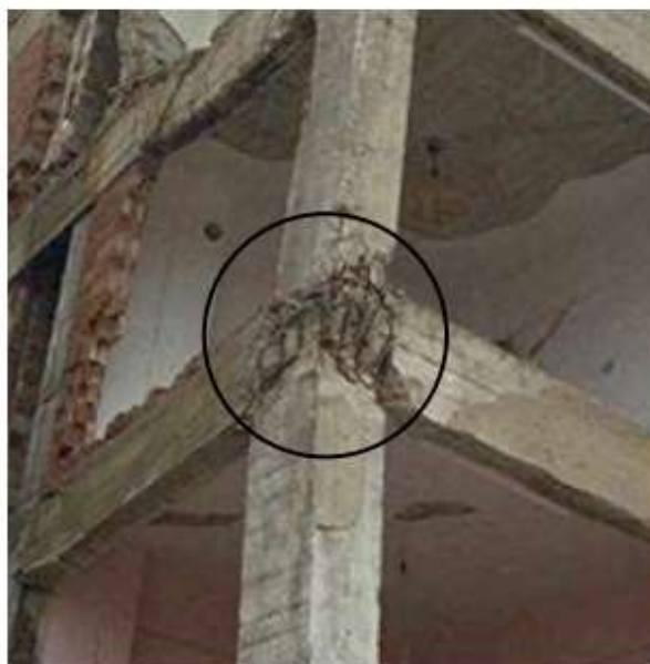
(b) Close-up of beam-column joint failure
