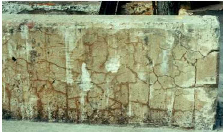
Fig. 5.3 Damage due to ASR on concrete
