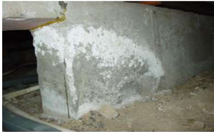
Fig. 5.4 Damage due to sulphate attack on concrete
