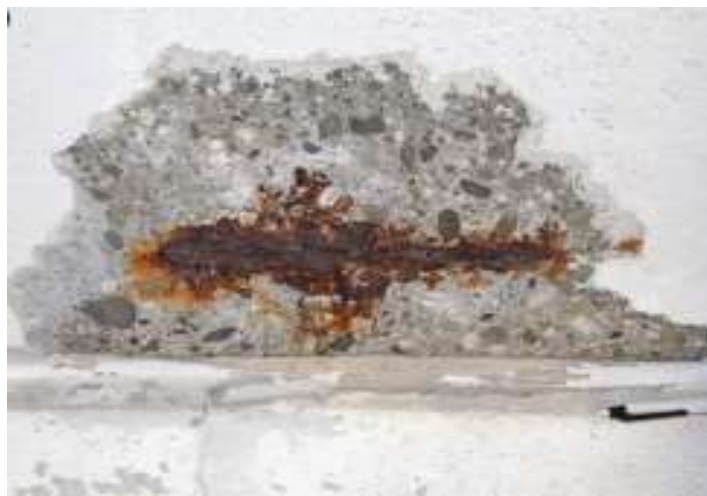
Fig. 5.2 Damage due to chloride attack on concrete
