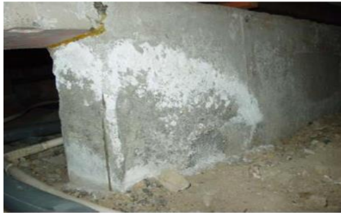
Fig. 5.4 Damage due to sulphate attack on concrete
