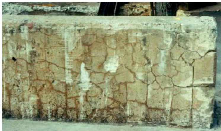
Fig. 5.3 Damage due to ASR on concrete
