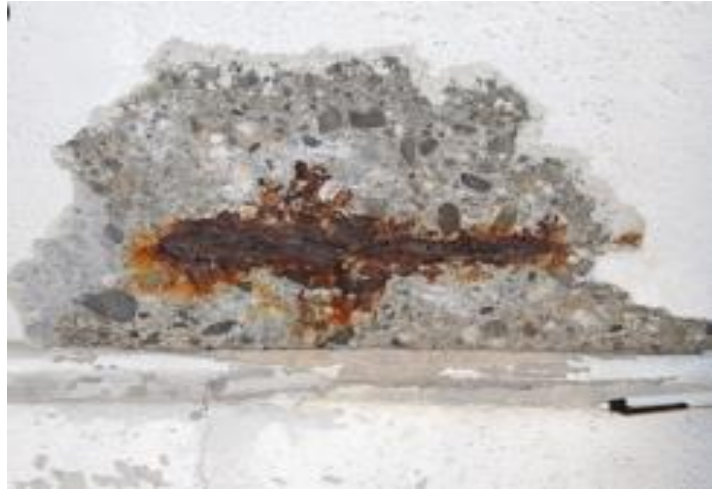
Fig. 5.2 Damage due to chloride attack on concrete
