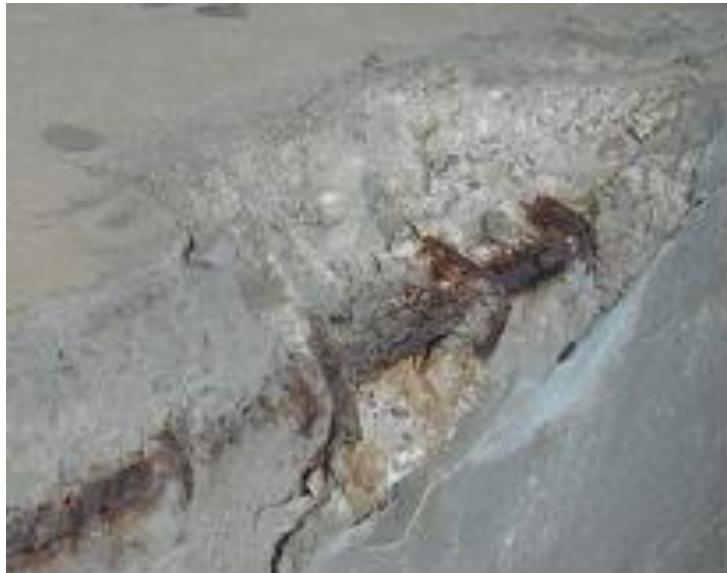
Fig. 5.1 Damage due to carbonation of concrete
