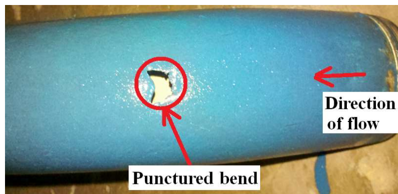
Fig. 1.9 Closer view of punctured pipe bend
