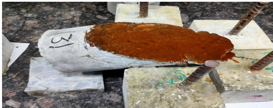
Fig. 4.13 Application of Epoxy to the inclined surface of Concrete for fixation of FRP sheet
