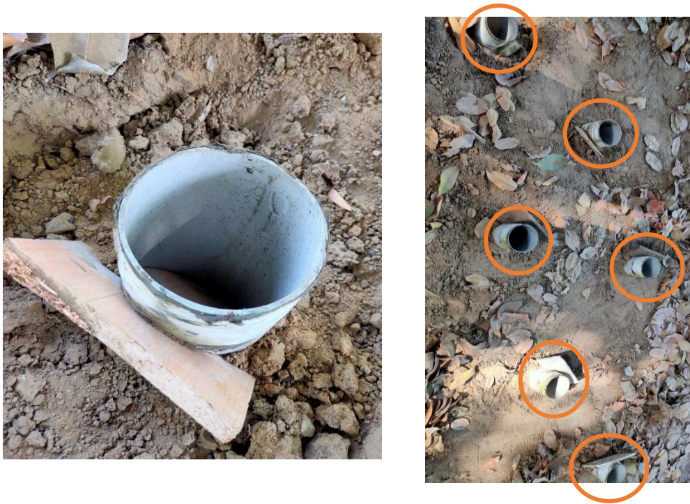
Fig. 4.7 Placing of molds in the pit with a flat plywood supported at the inclined surface
