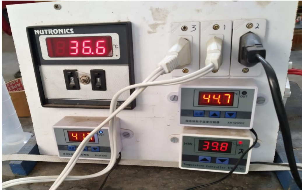
Fig. 3. 7 Temperature Control Panel
