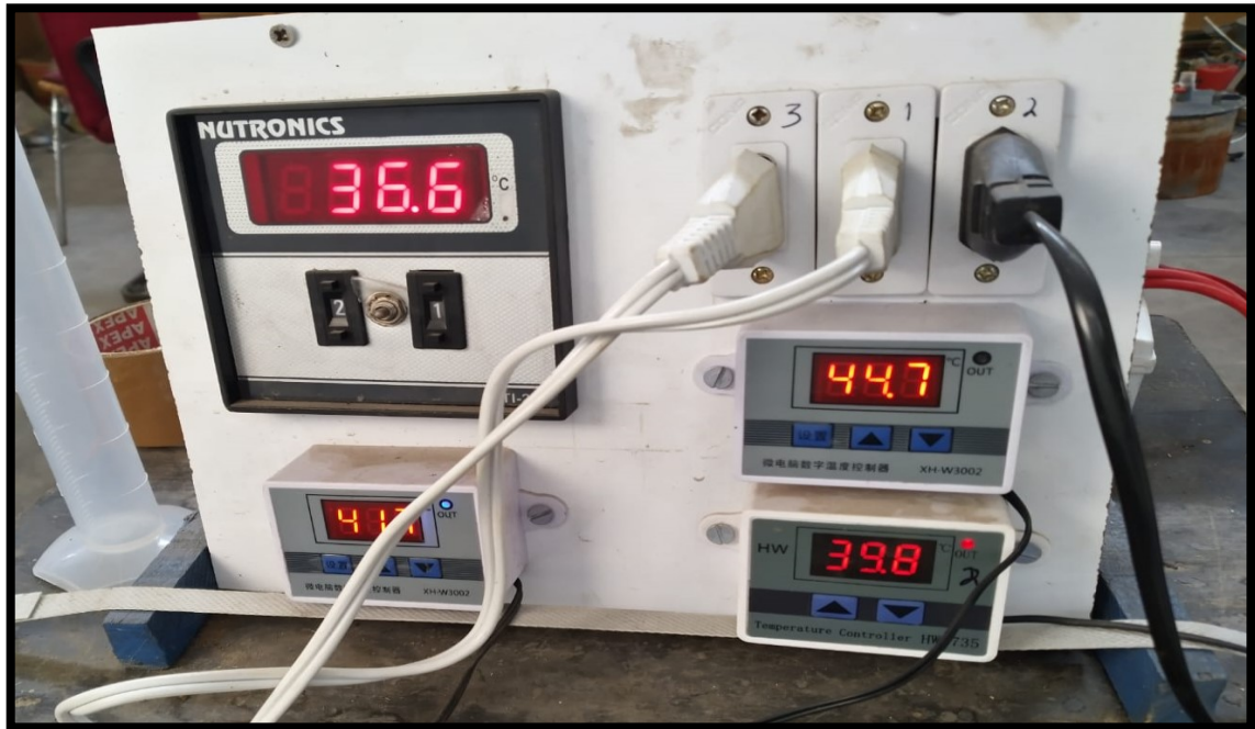
Figure 4.3: Temperature control unit
