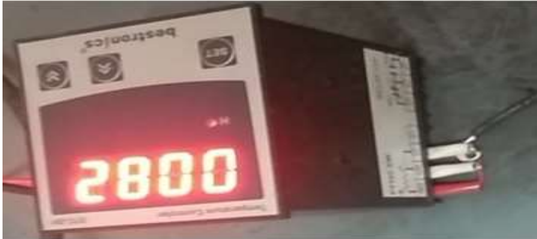
Fig.14: Thermocouple connected to display temperature reading
