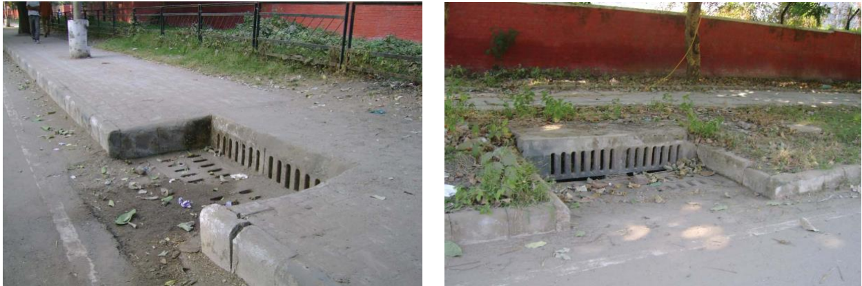
Figure 70: Stormwater Drain Inlet near the Road Capturing the Run-off from both Institutional Area (behind) as well as from Roads.
