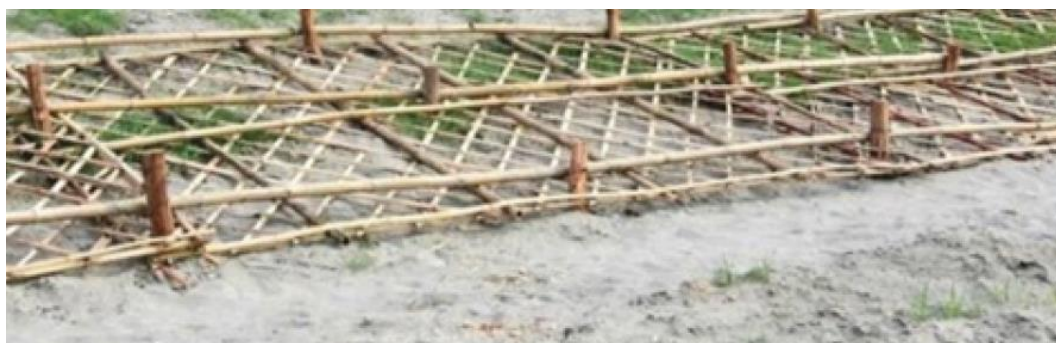
Figure 15: Top-Slope protection technique (Example: Concrete), Bottom- Bamboo sticks for slope protection, Bamboo Diameter was approximately 80mm, and number of mesh used were 405 nos.
