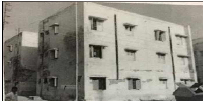
Figure 34: BHUJ: Stone in CM masonry building with minor damage
