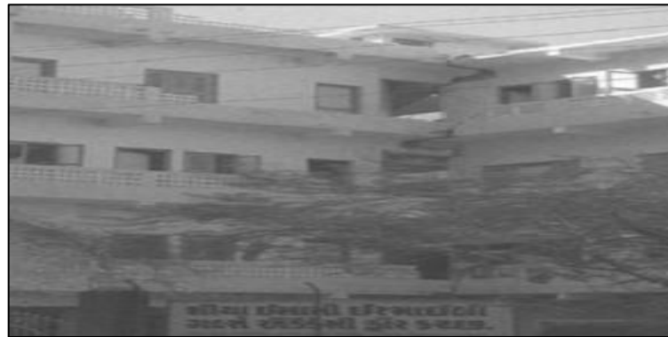
Figure 46: Damage to floor slabs and columns at the re-entrant corner of L-shaped building in bhuj
