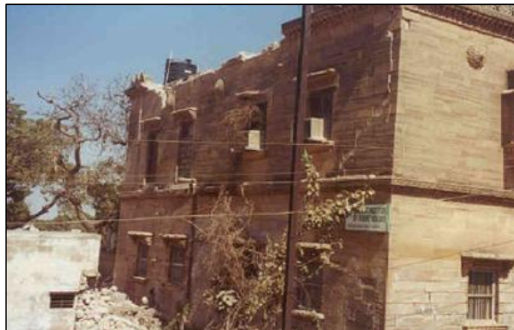
Figure 44: Cut-stone building in bhuj
