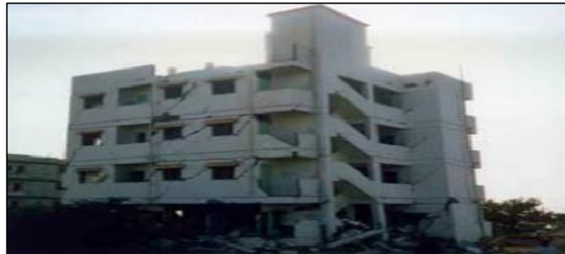
Figure 39: Soft storey collapse of a 5 storey apartment Building in bhuj
