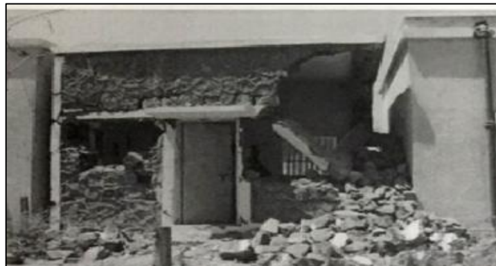
Figure 35: BHUJ: out of plane failure along with Lintel band failure.
