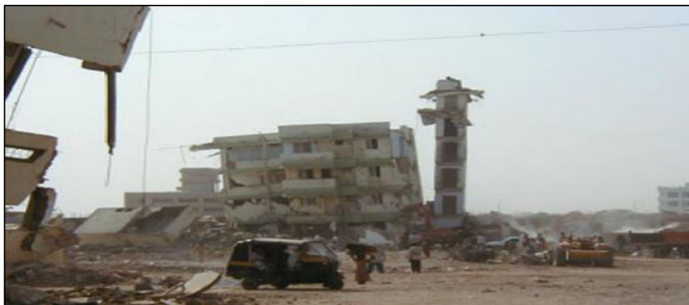
Figure 55: combination of collapses in Gandhidham
