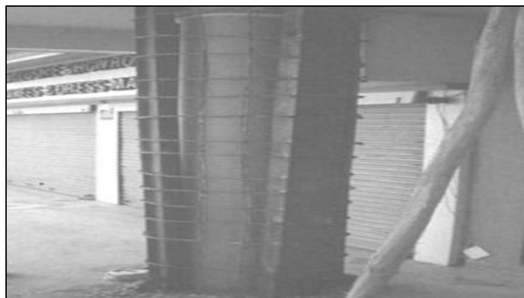
Figure 83: Hot-rolled I-sections were used to jacket the circular RC columns on the ground story of an 11-story commercial building in Ahmadabad. However, no connections were made between the steel I-sections and the concrete columns.
