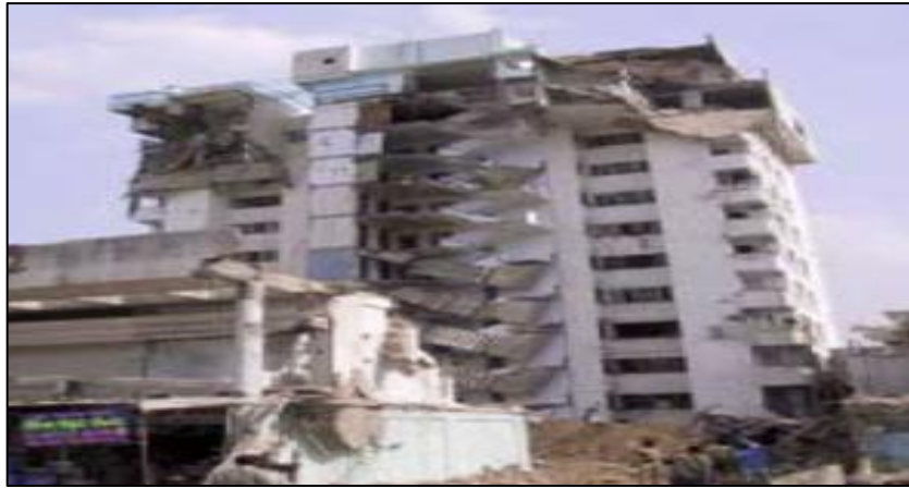
Figure 62: The 11-story building in front of Mansi Apartments, Ahmadabad collapsed due to a soft story. The presence of a swimming pool and reservoir at the top of the building added to the severity of the damage.
