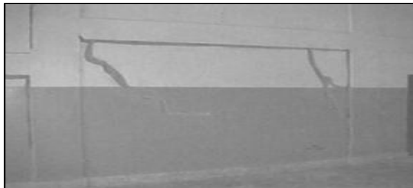
Figure 79: In the affected area, many buildings experienced frame-infill separation, which was fixed by cleaning and filling the gaps with rich cement mortar. The accompanying photo displays an example of this type of repair at a school building in Gandhidham
