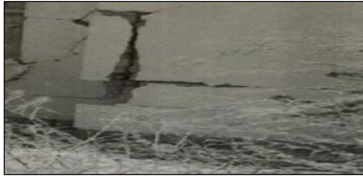
Figure 37: BHUJ: corner failure in the presence of corner reinforcement
