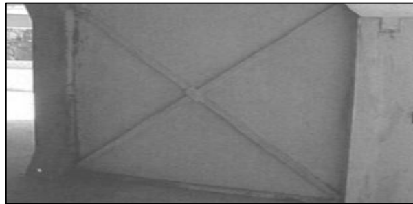
Figure 85: To reinforce open ground story panels, steel braces are used in specific cases. In this residential building, burnt clay brick masonry infill's were used to fill in the gaps, and steel sections were wedged at the outer faces. Additionally, steel hollow box sections with a size of 100 and a plate thickness of 8mm were used as bracing members.
