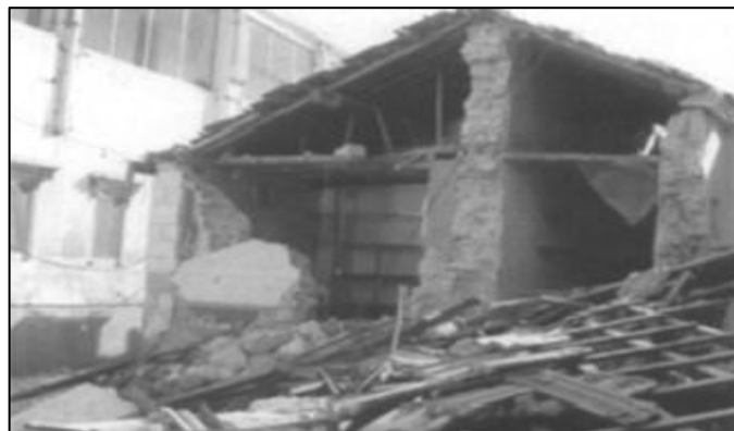
Figure 25: Damage to masonry construction due to inadequate connections between the walls
