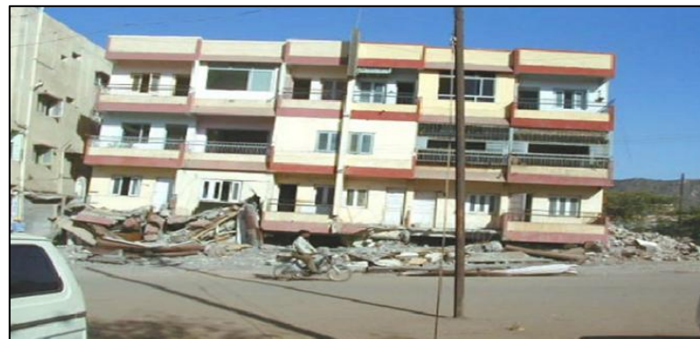
Figure 40: Typical soft storey collapse in Bhuj
