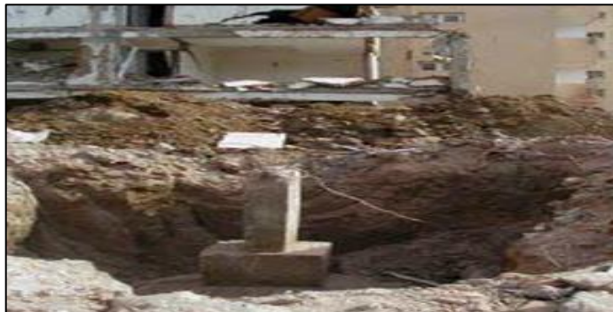
Figure 68: Column footing located approximately 2m below grade at Shikhar Apartments in Ahmedabad
