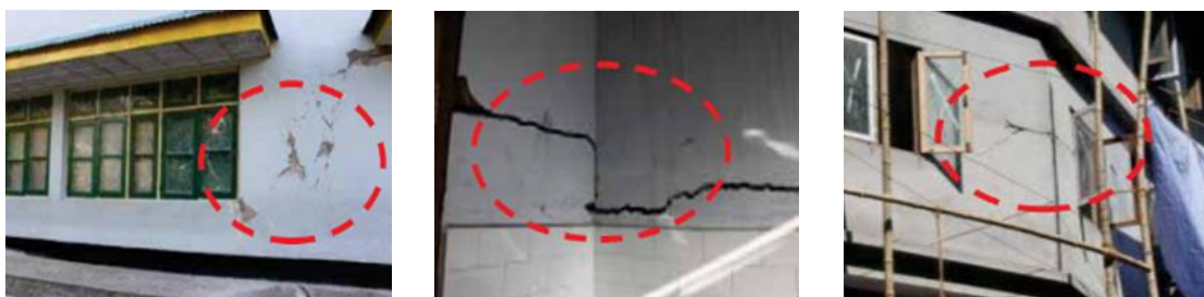
Figure 73: Damages in Unreinforced Masonry infill's
