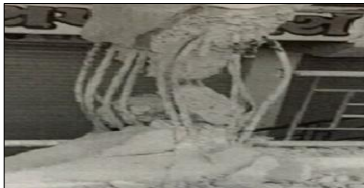
Figure 36: BHUJ: RC column failure
