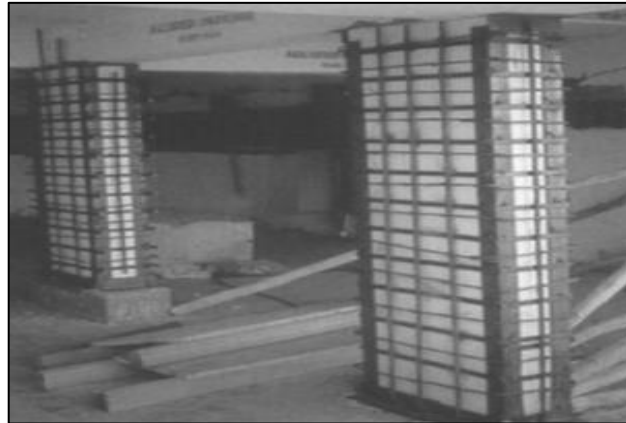
Figure 88: Before jacketing, mild steel angles measuring 75mm at four corners and 25mm steel flats were used as primary reinforcement for damaged RC columns in an open ground story building.
