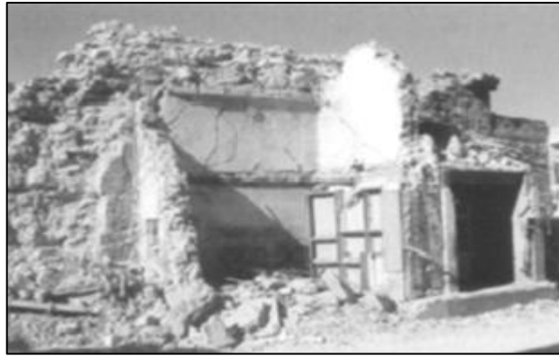
Figure 26: Damage to masonry construction due to inadequate connection between the walls
