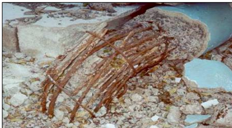
Figure 64: This image shows the reinforcement details of a column that failed in a soft storey collapse. It is apparent that the longitudinal bars are heavily congested due to their lapping at one location, and there are insufficient lateral ties over the splice length
