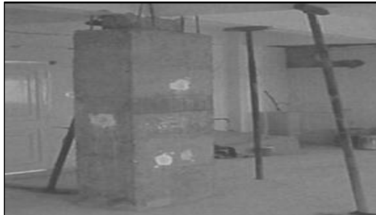
Figure 82: The ground level column of a seven-story old age home in Gandhidham was reinforced with a jacket, which covered it from the floor level to just below the top beams. In the visual, the column bars can be observed being curtailed on the side of the beam.
