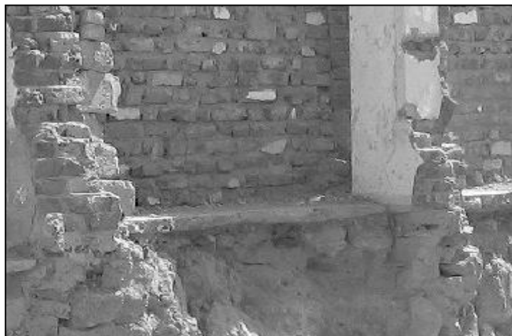
Figure 22: structure that is not designed. Before the earthquake, burned clay bricks and mud mortar were often used to build walls in Bachhau homes.
