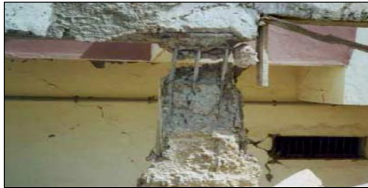
Figure 71: Poor quality concrete and lack of seismic detailing evident in beam column connection
