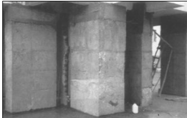
Figure 89: The original purpose of open ground stories in RC frame buildings was for parking, but after reinforcing the columns with jackets, the available space for cars was limited due to increased column size, leading to a disruption of the intended parking function.
