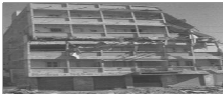
Figure 48: Intermediate story collapse in the 6 story building in Bhuj
