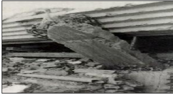
Figure 50: Gandhidham: Column failure – shaking in weaker direction
