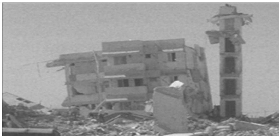
Figure 57: Incorrect attachment to RC elevator core walls in Gandhidham.
