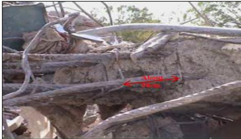
Figure 63: This image provides a detailed look at the debris of Mansi complex, revealing the placement of reinforcement and the quality of concrete used in the collapsed columns.
