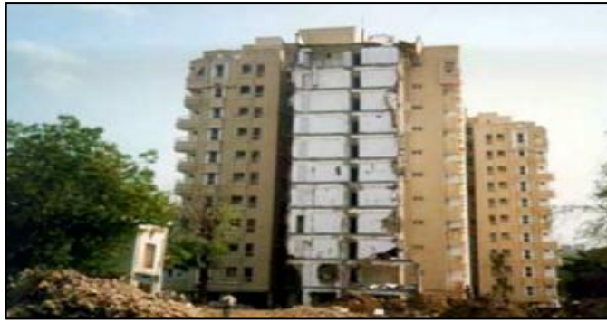
Figure 67: Shikhar apartments, Ahmadabad .Building collapsed due to soft story effects
