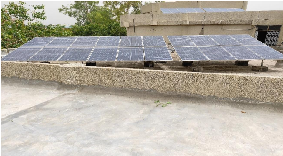
Fig. 4.1: - 5 kW Photovoltaic System
