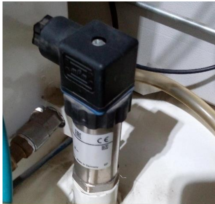
Plate 3.12: Air flow sensor
