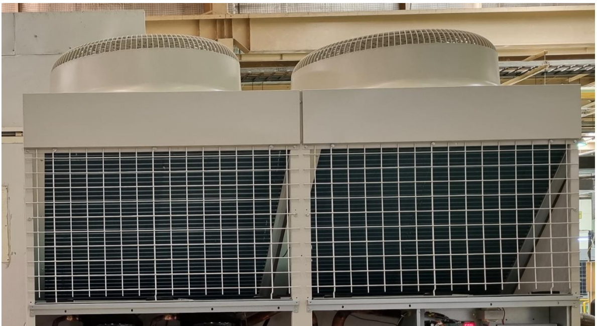
Figure 1.13.1 Air Cooled Condenser [19]
