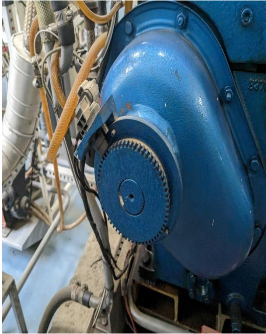
Figure 3.2.3 Engine speed measurement device
