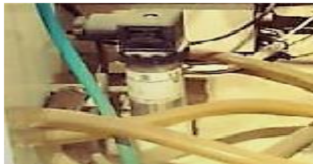
Plate 3.22 Air flow sensor
