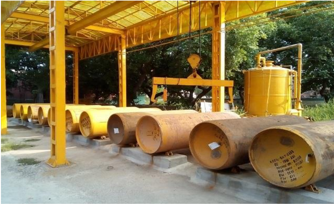
Figure 7: Chlorination system of Water at a Water Treatment Plant in Delhi
