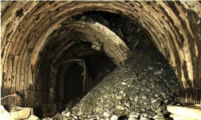
Fig 1.4 Photograph of the collapse in the tunnel extending towards the face (Source: Google image)
