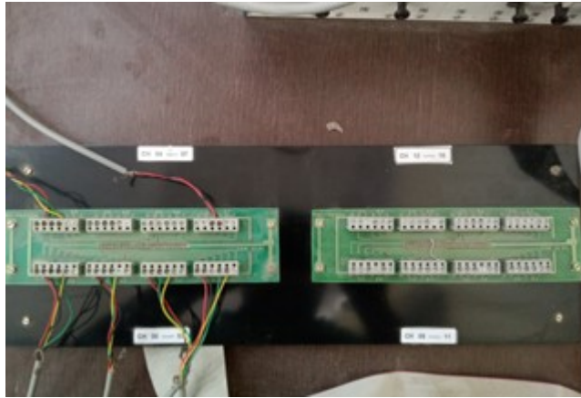
Fig. 3.8 16-Channel Plate attached with LVDT Data acquisition system
