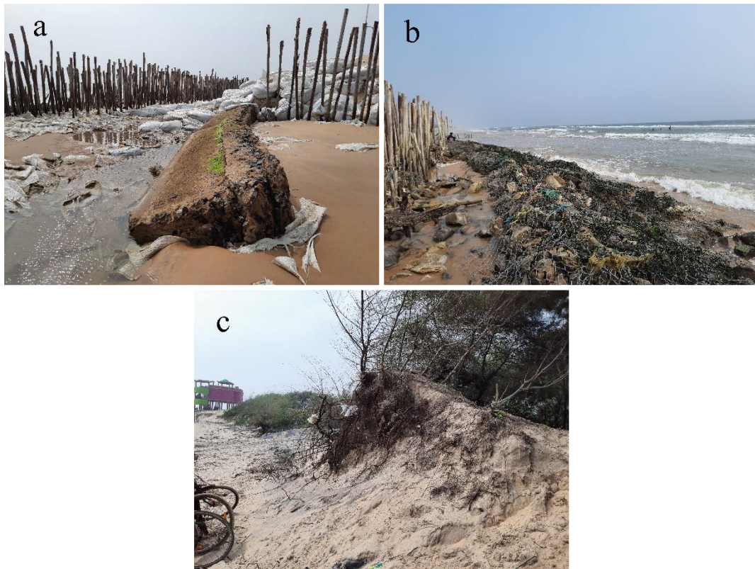
Figure 4.4 a. The breakwater structures, b. the concrete sea walls, c. at the Siali beach of Ersama block
