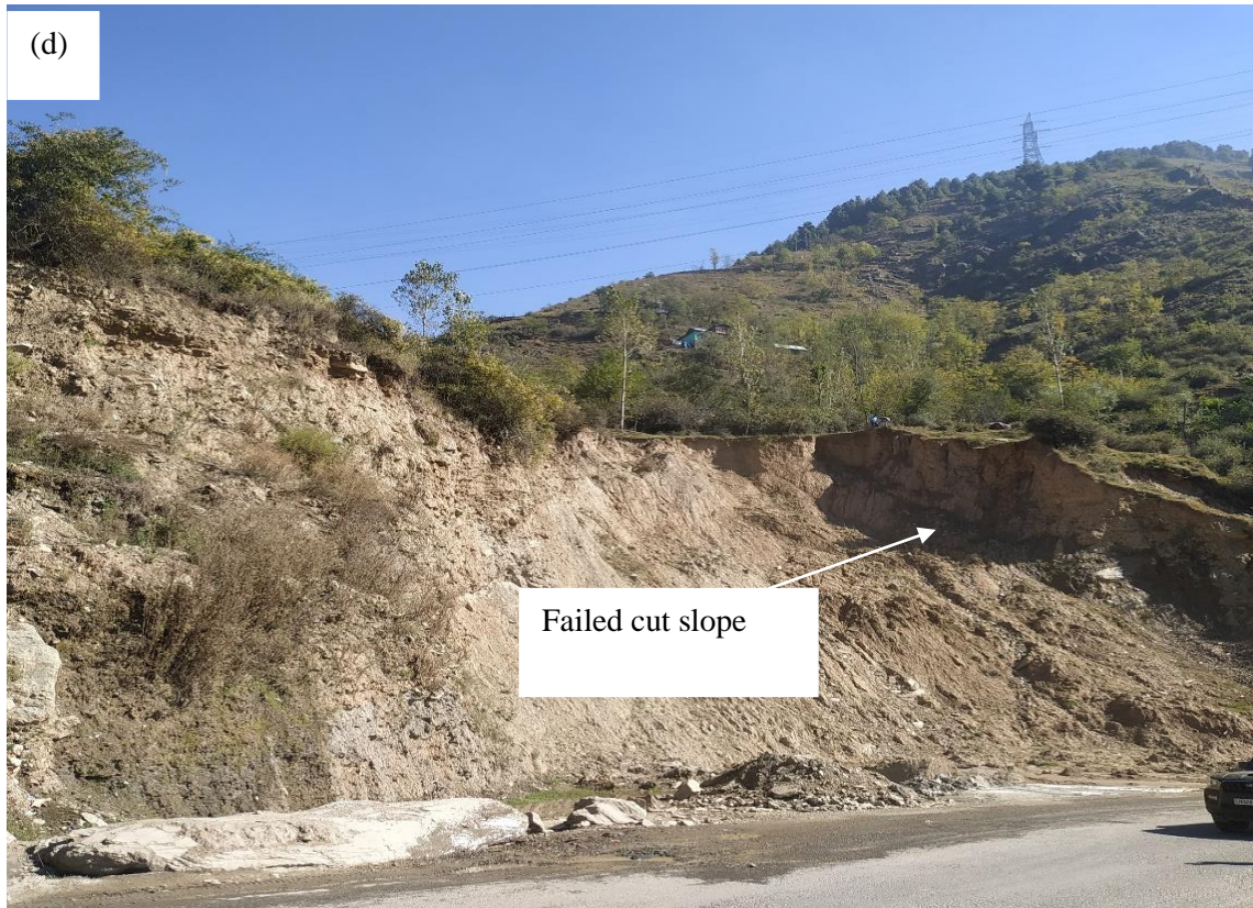
Fig. 1.2: Pictures showing (a) Intercepted water along road (b) Steep cut slope along road (c) slopes under possible progressive failure (d) Failed cut slope along road
