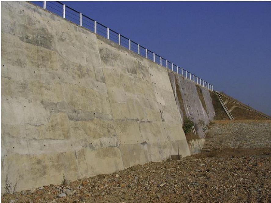
Figure 1.1 The geogrid supported soil retaining wall's front face has a cast-in-place concrete-rigid facing. (G. Yang et al. 2009)
