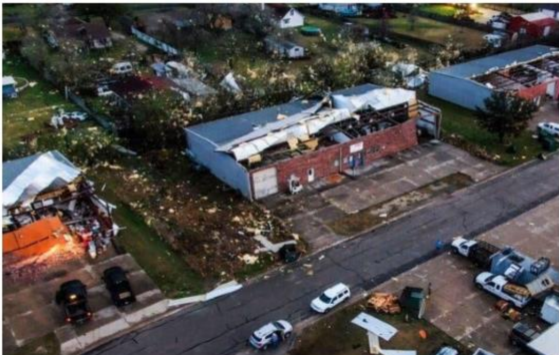
Fig. 1.2 Aerial view of damaged roofs due to high-speed wind in Texas, 2022.
