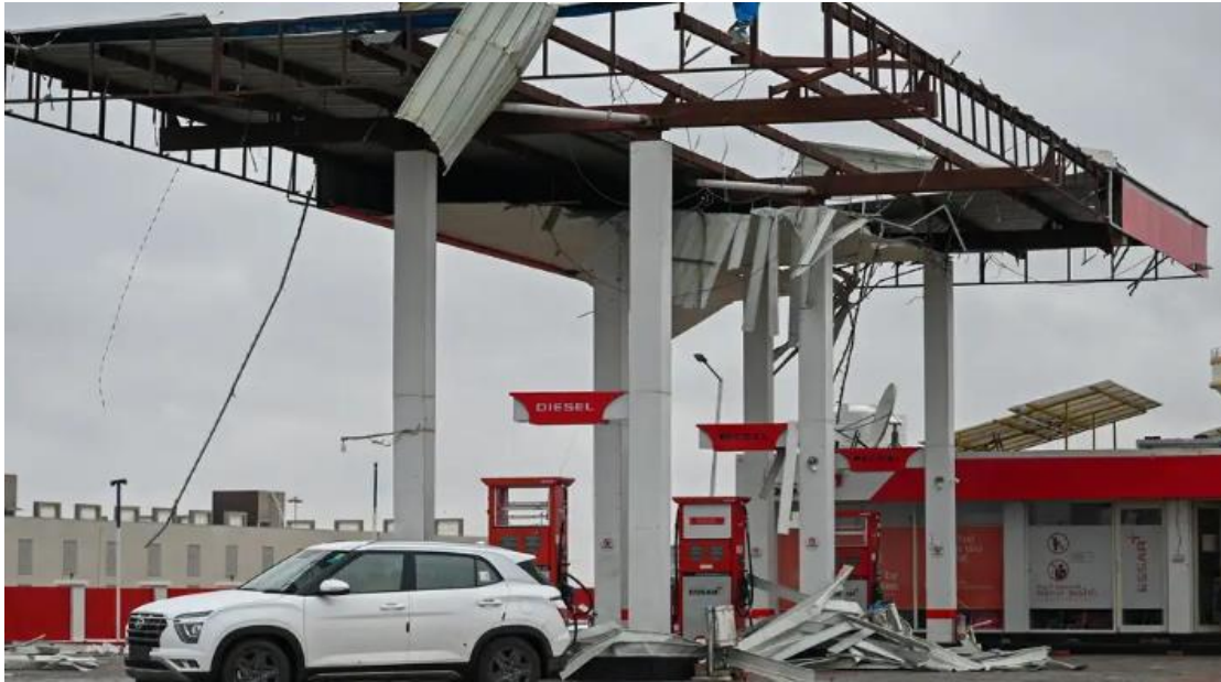
Fig.1.1 A damaged fuel station can be seen after the impact of Cyclone Tauktae near Amreli on May 18, 2021. (Punit Paranjpe/AFP via Getty Images)
