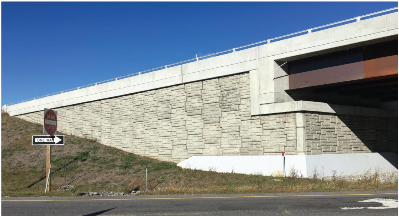
Figure 1.2 Use of Lower GRS Wall in Narayanapuram Road bridge, Chebrolu (Andhra Pradesh)
