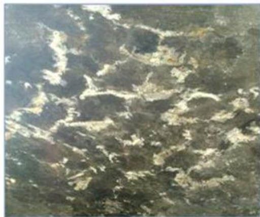
Fig 3.6 Leaching observed in soffit slab
