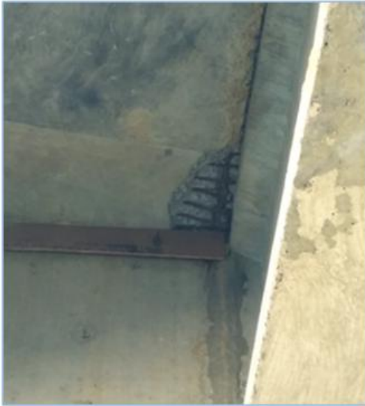
Fig 3.3 Exposed Reinforcement Observed in deck slab
