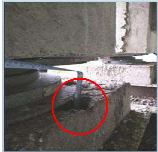
Fig 3.17 Cavity observed under the bearing plate at pedestal
