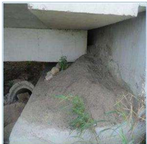
Fig 3.35 Debris accumulated around the bearing, affected the performance of bearings.
