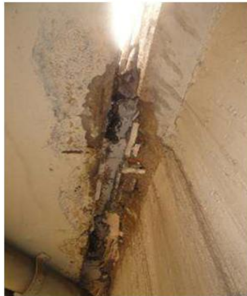
Fig 3.15 Underside portion of expansion joint severely damaged
