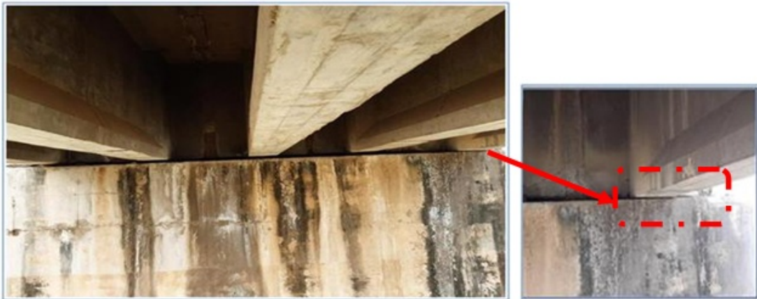
Fig.4.1 Out of five Girders one girder resting on pier cap without bearing
