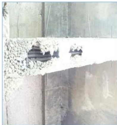
Fig 3.60 Exposed reinforcement at bottom of diaphragm
