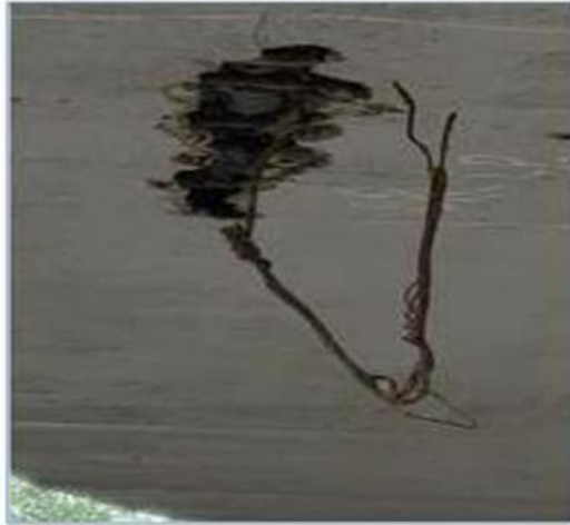
Fig 3.1 Exposed Reinforcement and also seen unwanted material in deck slab
