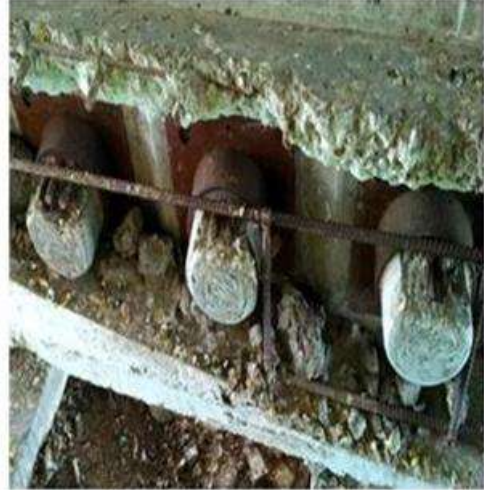
Fig 3.40 Prestressing cables exposed at end girder
