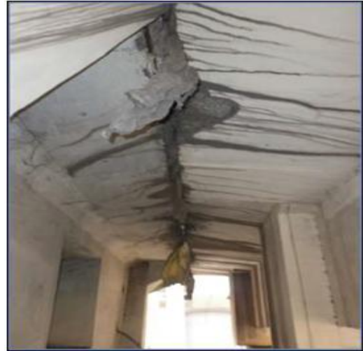
Fig 3.14 Underside portion of expansion joint damaged
