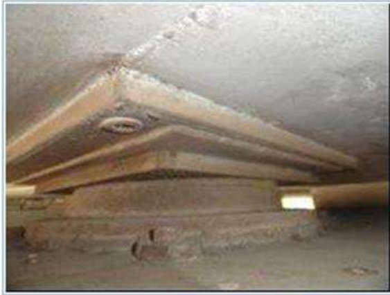
Fig 3.30 bolts are missing in bearing plate
