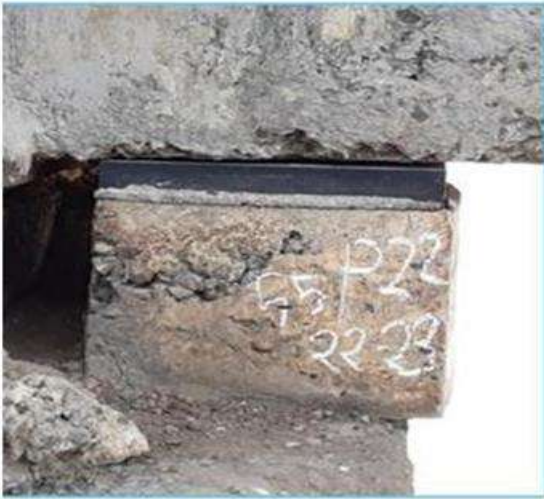
Fig 3.16 Pedestal not casted properly
