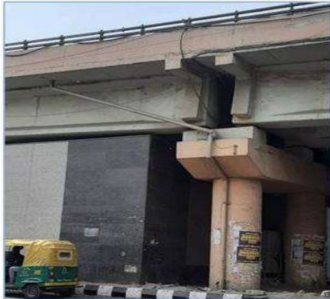
Fig 3.55 Proper down take pipe provided.
