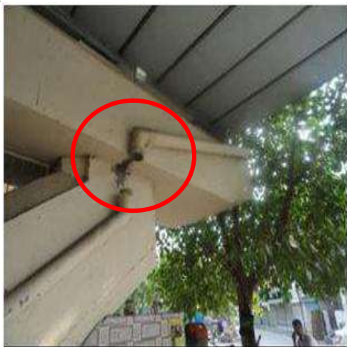
Fig 3.57 It shows Drainage pipe provided properly but got damaged and it has not been noticed due to lacking of inspection.
