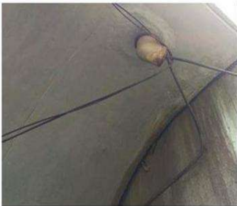
Fig 3.49 Improper down take pipe
