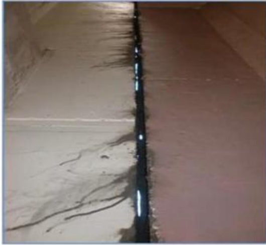
Fig 3.13 Neoprene seal missing in expansion joint and water leakage observed
