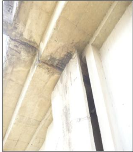
Fig 3.4 Exposed Reinforcement Observed in cantilever portion
