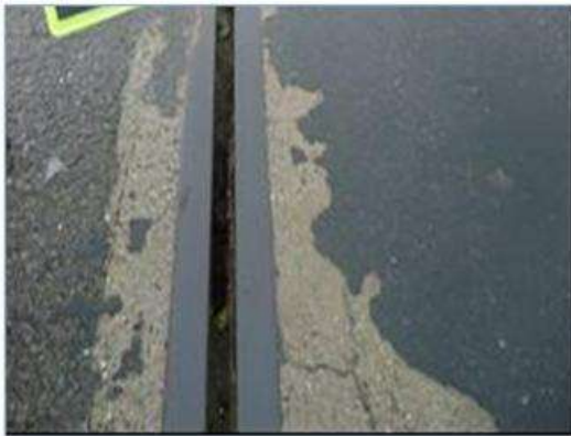
Fig 3.9 Neoprene seal missing in expansion joint due to movement affected
