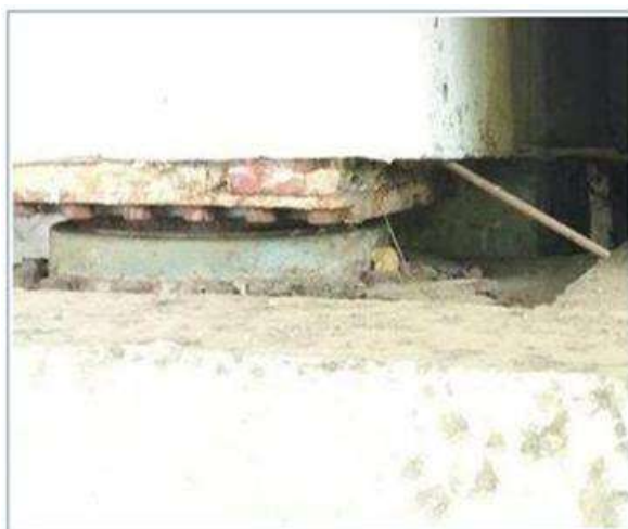
Fig 3.34 Unwanted R/F bar exposed
