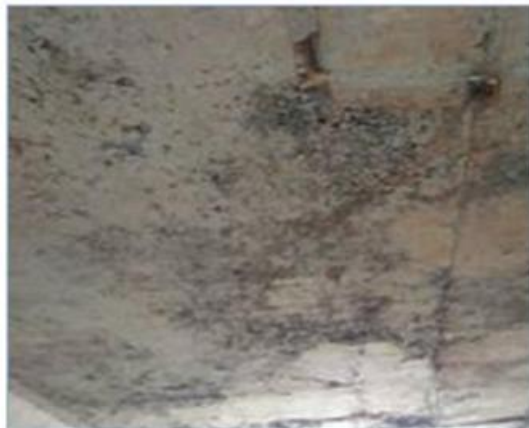
Fig 3.5 Honeycombing observed in soffit Slab
