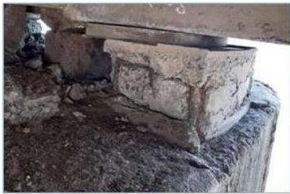
Fig 3.26 Bearings not placed properly
