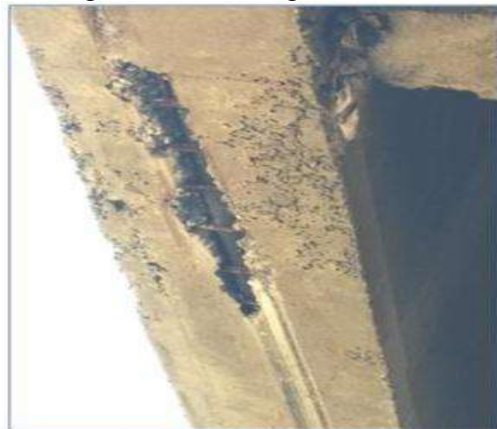
Fig 3.43 Exposed sheathing as seen from the bottom in the bottom flange of girder
