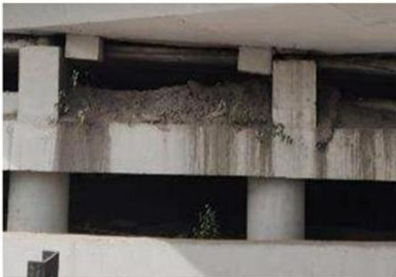
Fig 3.22 Debris accumulated over the pier cap
