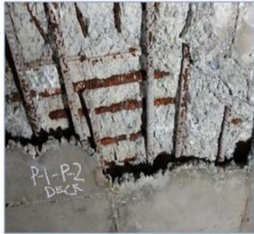
Fig 3.2 Exposed Reinforcement Observed in deck slab
