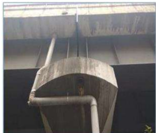
Fig 3.19 Seepage on pier cap
