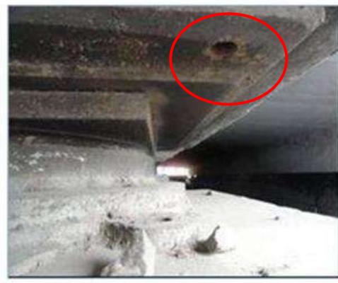
Fig 3.29 bolts are missing in bearing plate
