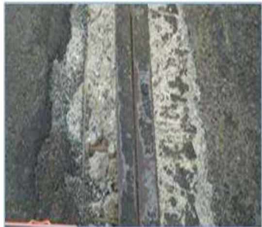
Fig 3.12 Exposed reinforcement in edge beam of expansion joint
