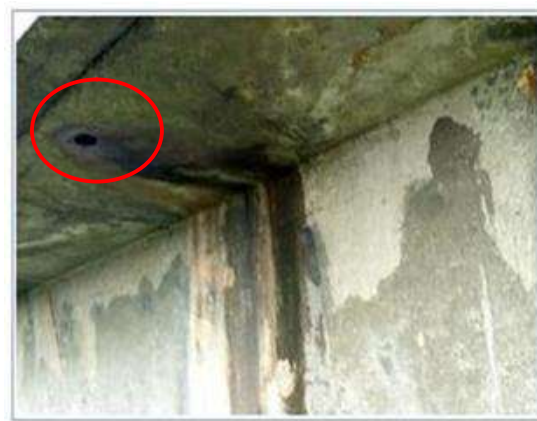
Fig 3.52 Seepage observed on structure surface due to improper drainage system
