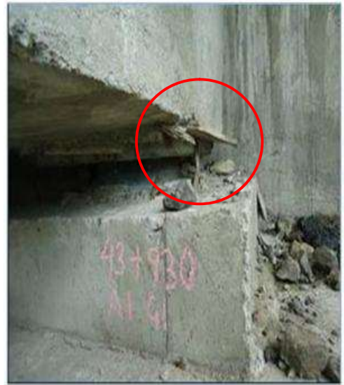
Fig 3.33 Locked bearing is observed as sleeves are not opened for free movement
