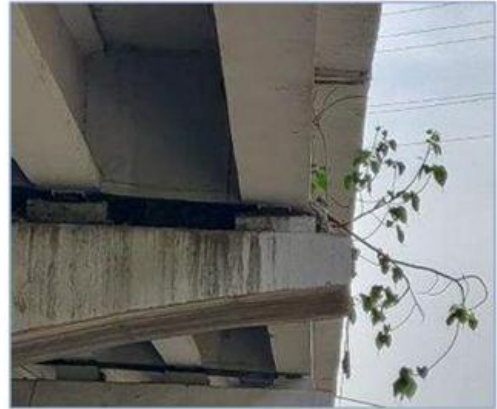
Fig 3.21 Vegetation growth on pier cap
