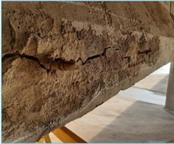
Fig 3.45 Poor repair work
