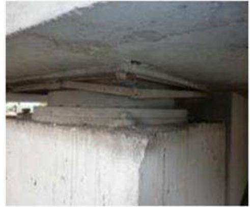
Fig 3.31 Bearing steel plate damaged
