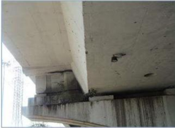
Fig 3.20 Vegetation growth on pier cap
