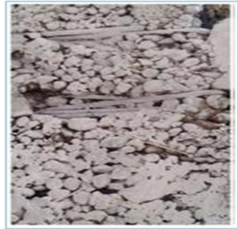
Fig 3.46 Honeycombing as seen at the bottom of the flange of girder
