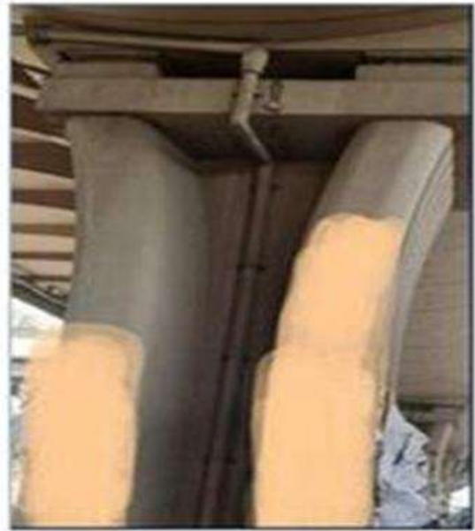
Fig 3.54 Proper down take pipe provided.
