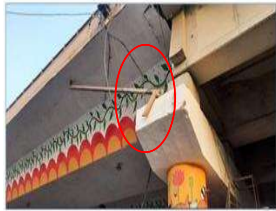
Fig 3.56 Improper down take pipe provided
