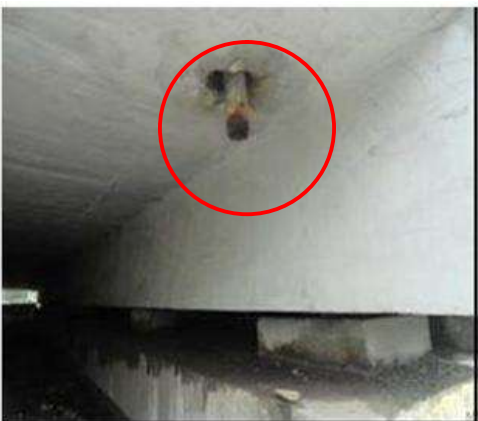
Fig 3.51 Improper down take pipe
