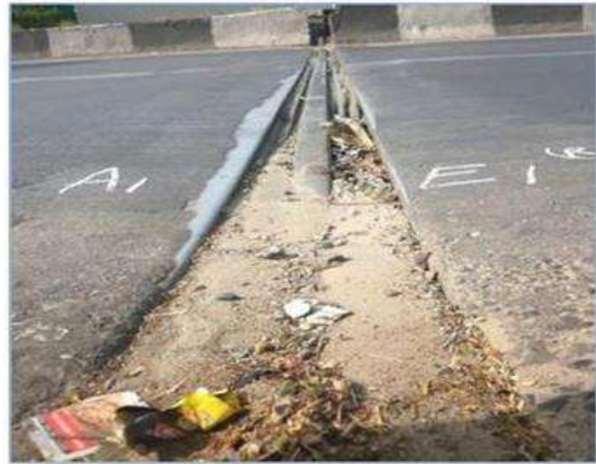
Fig 3.8 Debris accumulated in expansion Joint
