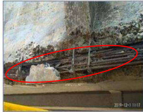
Fig 3.42 Prestressing cables corroded
