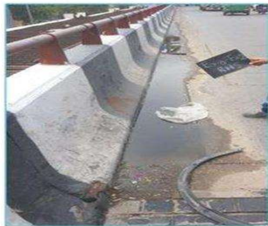
Fig 3.58 Water logging observed at road level
