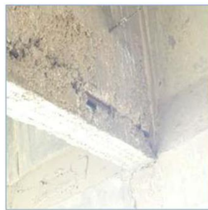
Fig 3.61 Exposed reinforcement in the face of diaphragm
