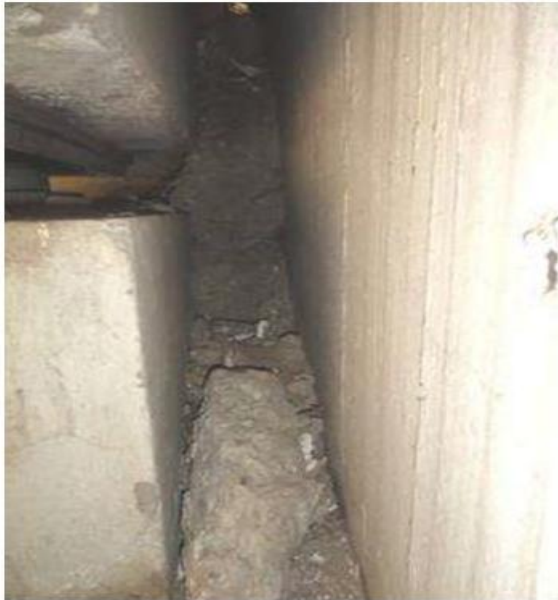
Fig 3.24 Concrete accumulated at pier cap due to negligence during the construction
