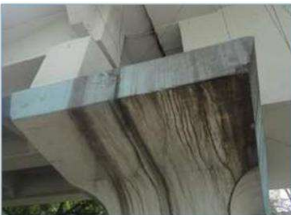
Fig 3.18 Seepage on pier cap
