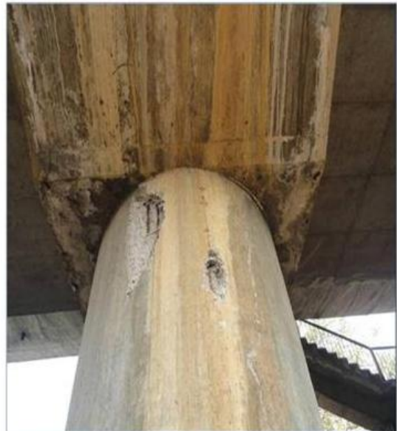
Fig 3.48 Exposed reinforcement observed on pier
