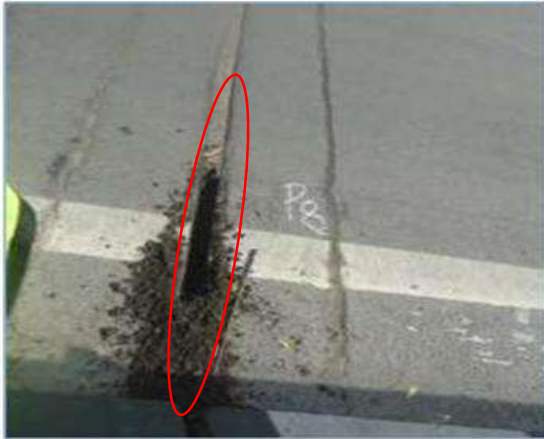
Fig 3.7 Debris accumulated in expansion joint
