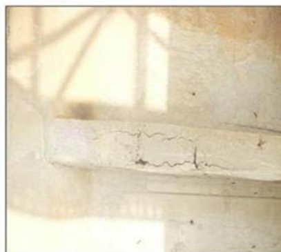
Fig 3.62 cracks observed at the bottom of diaphragm
