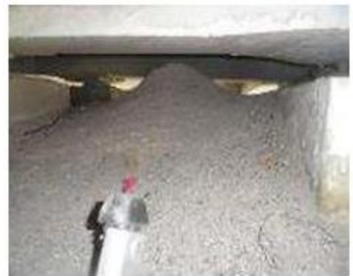
Fig 3.23 Debris accumulated over the pier cap
