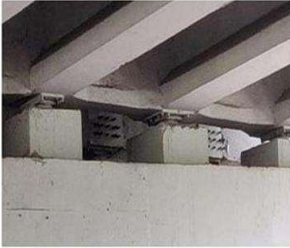
Fig 3.39 Prestressing cables exposed at end girder
