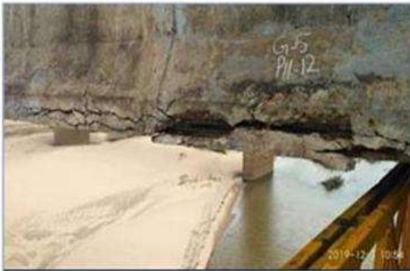
Fig 3.41 Prestressing cables corroded
