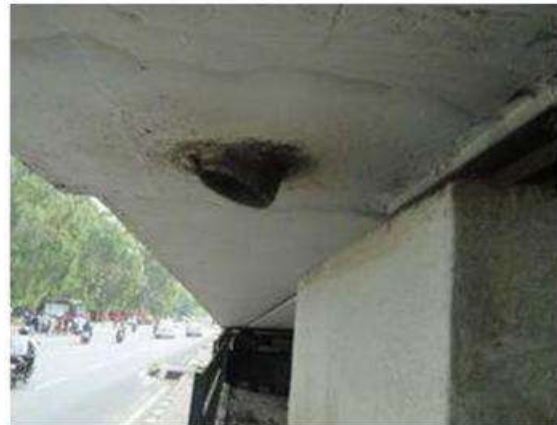
Fig 3.50 Improper down take pipe
