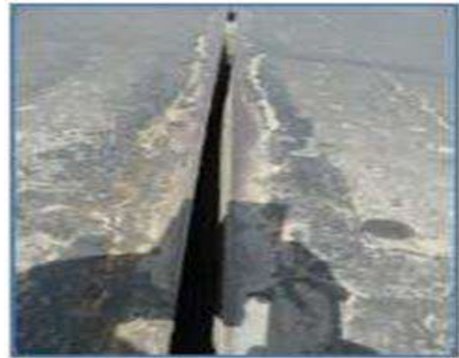
Fig 3.10 Neoprene seal missing in expansion joint due to movement affected
