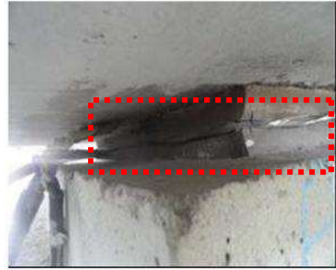
Fig 3.37 cuts on bearing is observed
