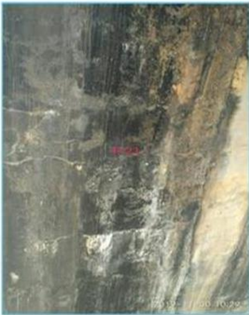
Fig 3.47 Leaching observed on pier
