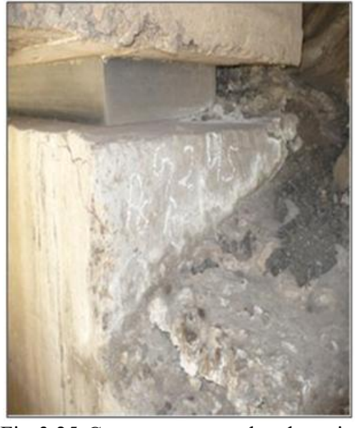
Fig 3.25 Concrete accumulated at pier cap due to negligence during the construction
