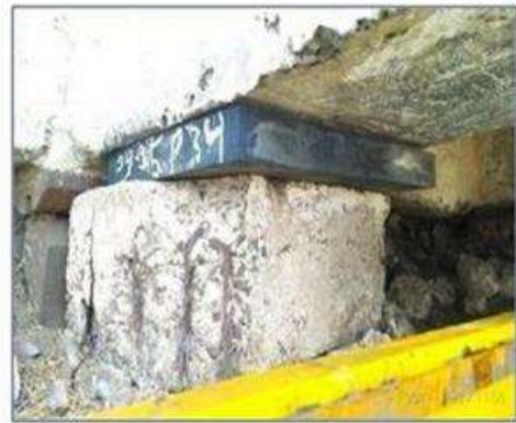
Fig 3.27 Bearings not placed properly
