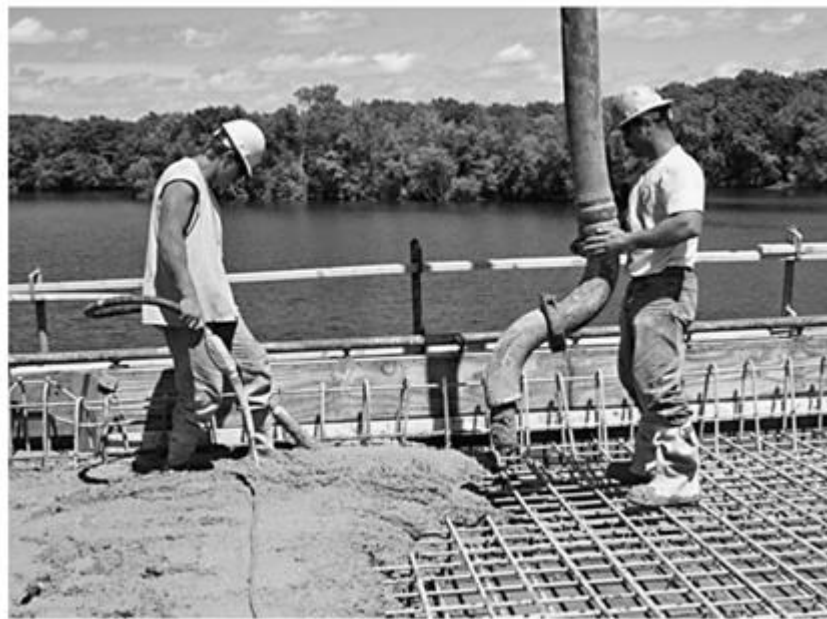
Figure 1: Workers placing and vibrating concrete on a bridge deck including epoxy-coated reinforcing steel. (Portland Cement Association) [1]
