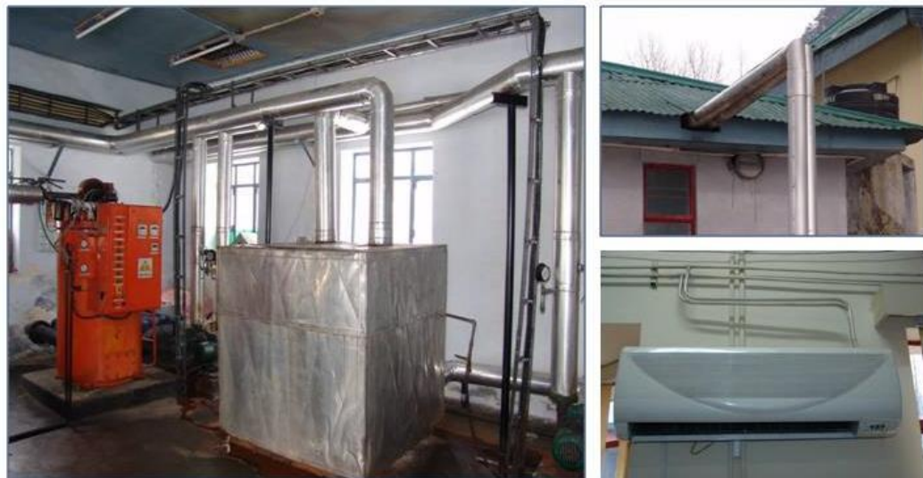
Figure 4.1: Performance evaluation of GSHP based space heating system with existing central heating plant connected to the dwellings.
