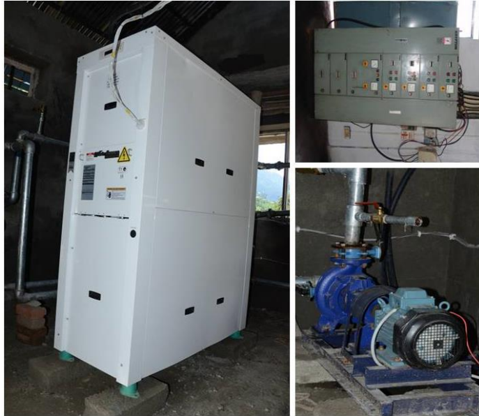
Figure 3.8: The Ground Source Heat Pump installed at the project site along with its control panel (right side top) and circulating pump (right side bottom).
