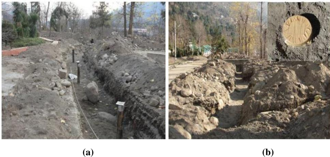
Figure 3.3: (a) The drilled boreholes as shown by uncut top portion of MS-casing in trench, (b) the top cut view of covered borehole and trench after cutting top portion of the MS-casing (ready for installation of U-bent).
