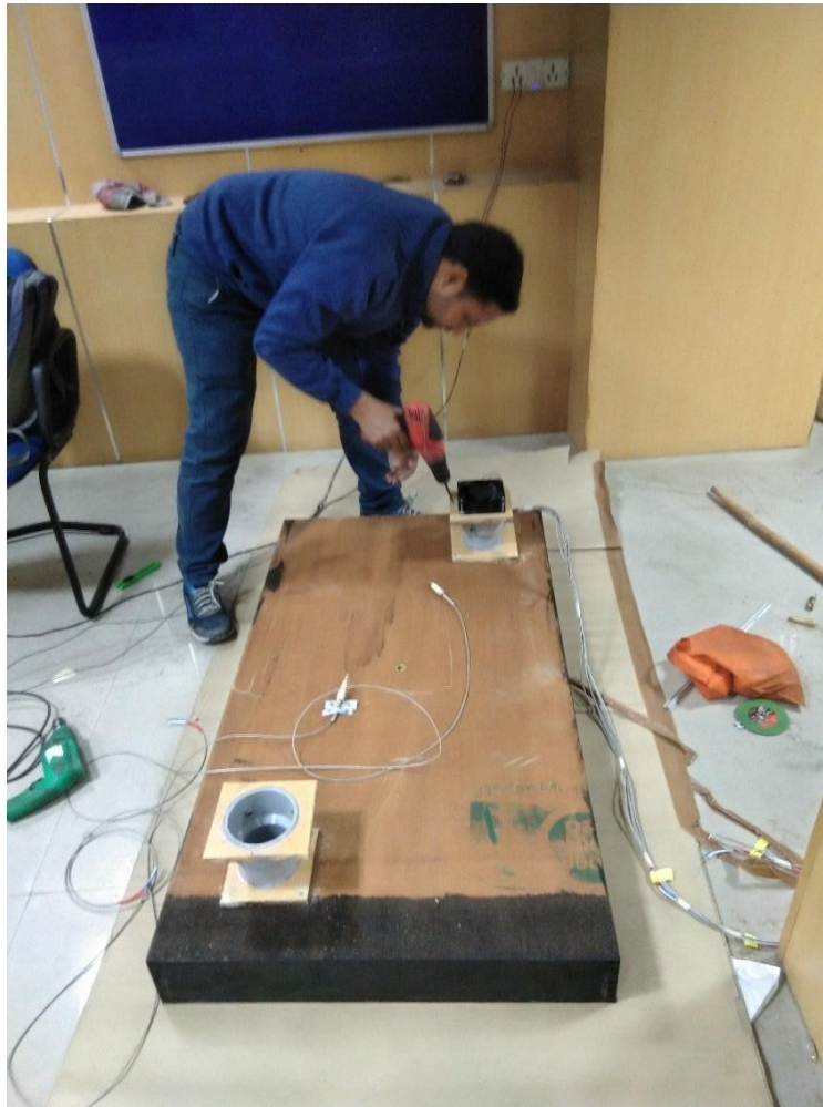
Figure 4.1.7: Installation of fan at the inlet of wire mesh collector
