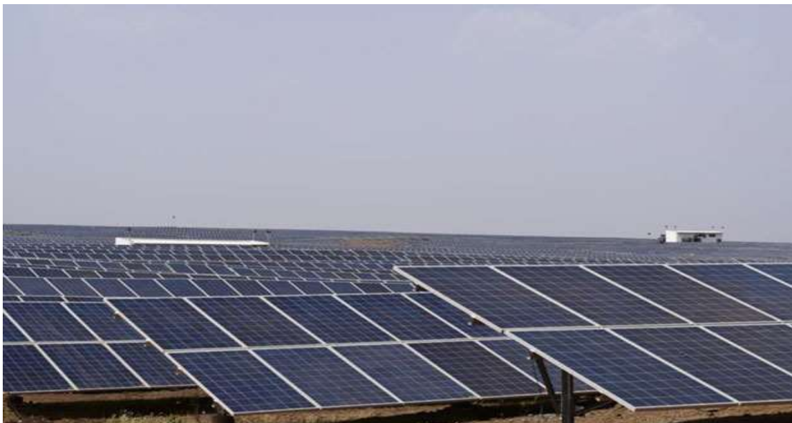
Fig.1.1 REWA solar power plant
