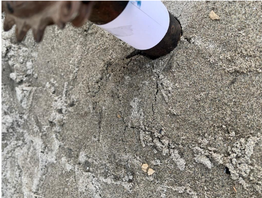
Figure 14 Crack occurred due to torsion
