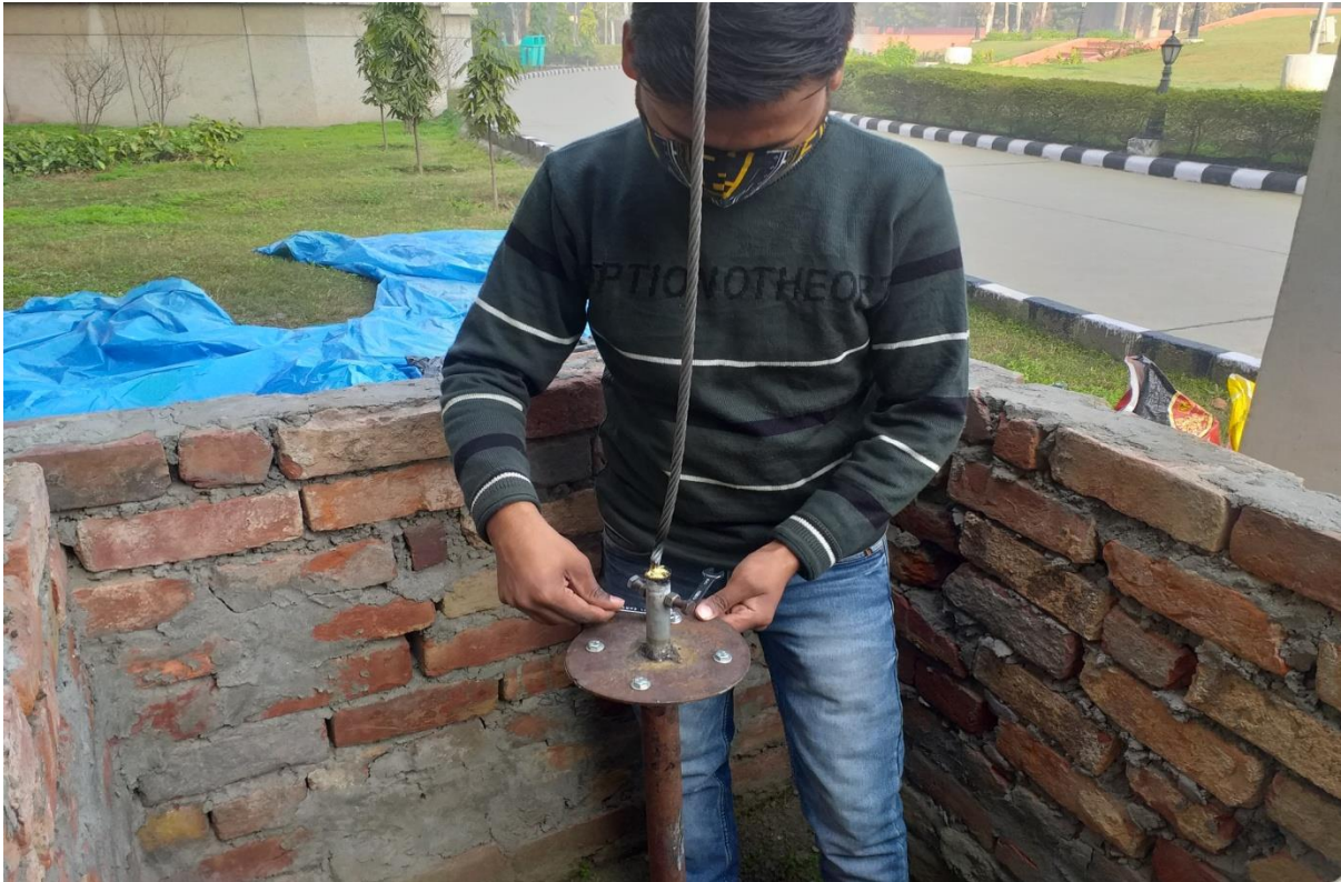
Fig.3.18 connection of both circular plates with the help of nut and bolts (By myself)
