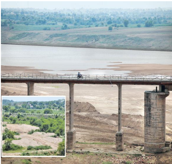
Figure 3.4 Erosion at bridge foundation
