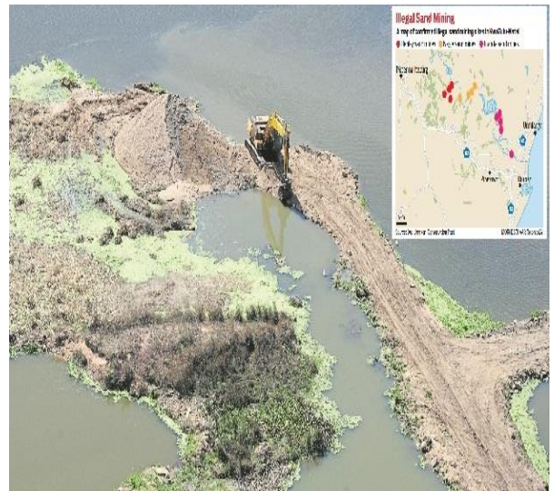
Figure 3.5 Road created for sand mining
