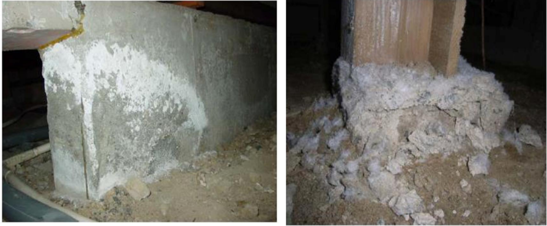
Figure 2: Sulphate attack in concrete
