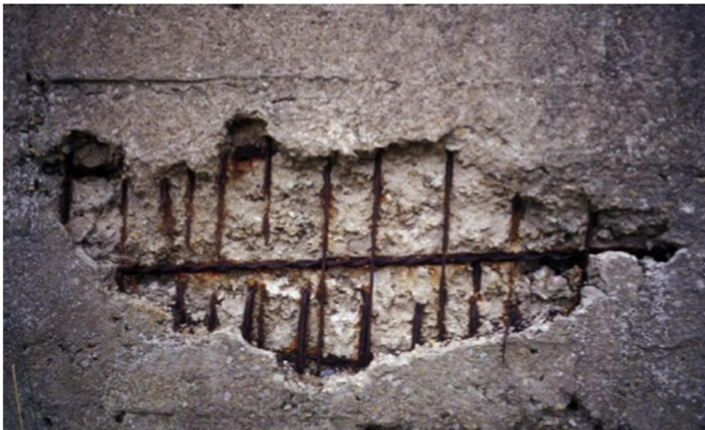
Figure 3: Chloride attack in concrete
