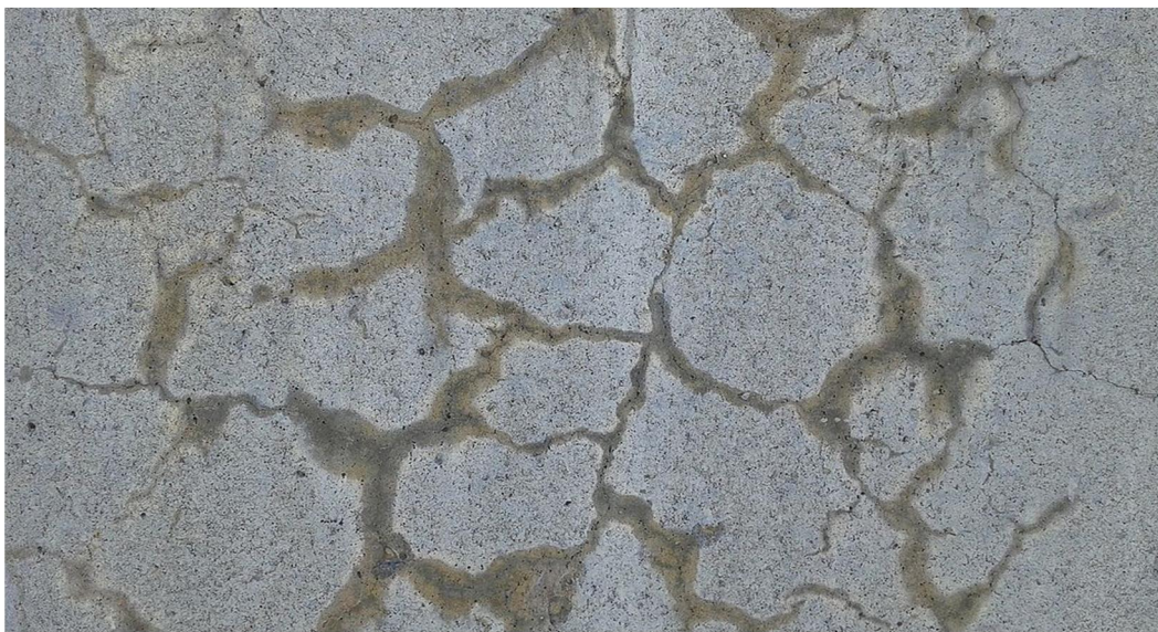
Figure 1: Alkali Silica reaction in Concrete
