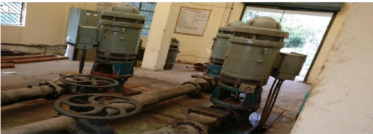
Fig.11: Sewage sample site and sewage pump house
