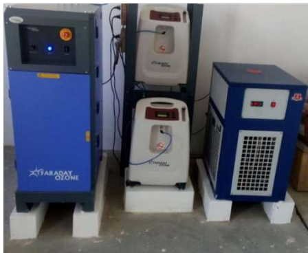
Figure 4.15 Showing Ozonation system as a downstream process for water recovery.
