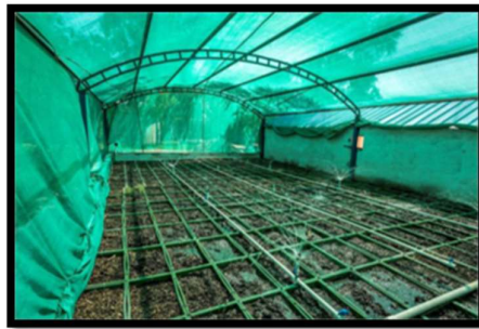
Figure 4.17 Showing civil based Bio-filter (for larger capacity)
