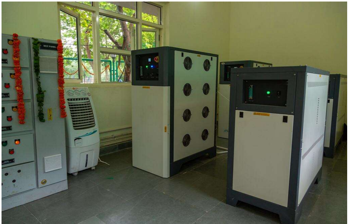
Picture-6 Ozonator System for Effective Disinfection
