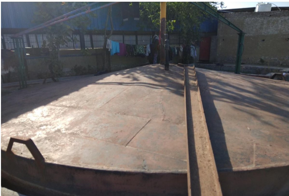
Figure 8.7: Shri Krishna Gaushala Biogas Plant Digester
