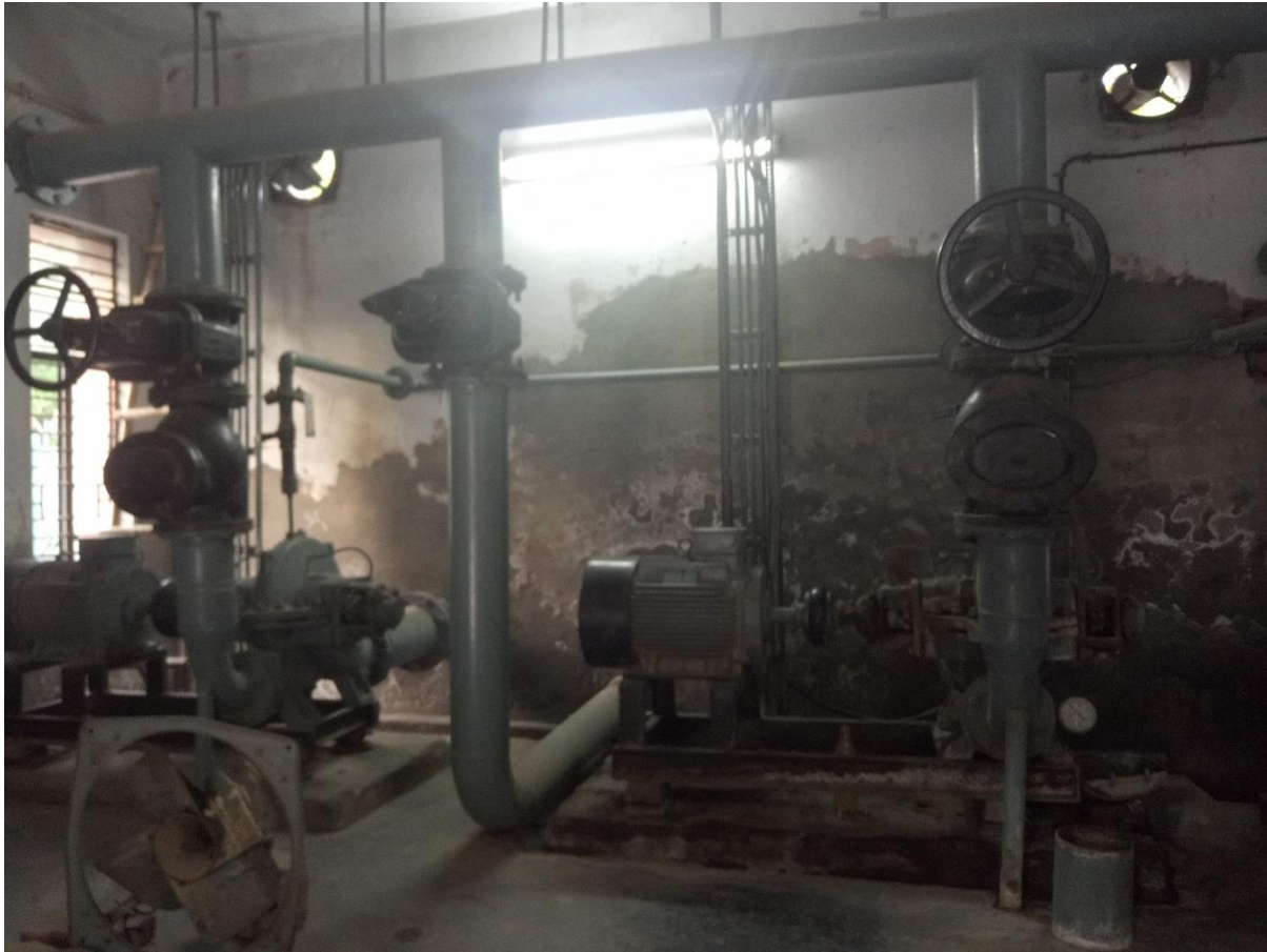
Figure 1 3: Water Pumping House
