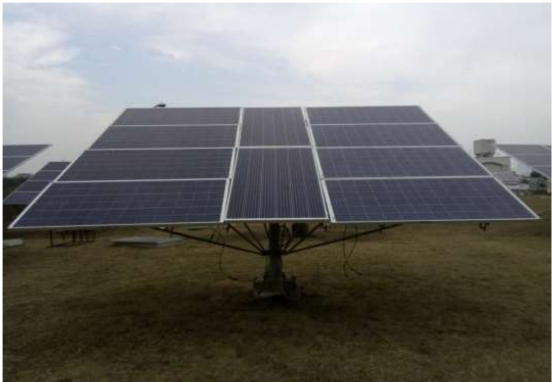
Fig. A.2 Experimental demonstration of multi-crystalline solar PV module at National Institute of Solar Energy (NISE), India
