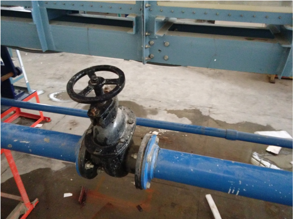
Figure 4.2 Valve for controlling discharge
