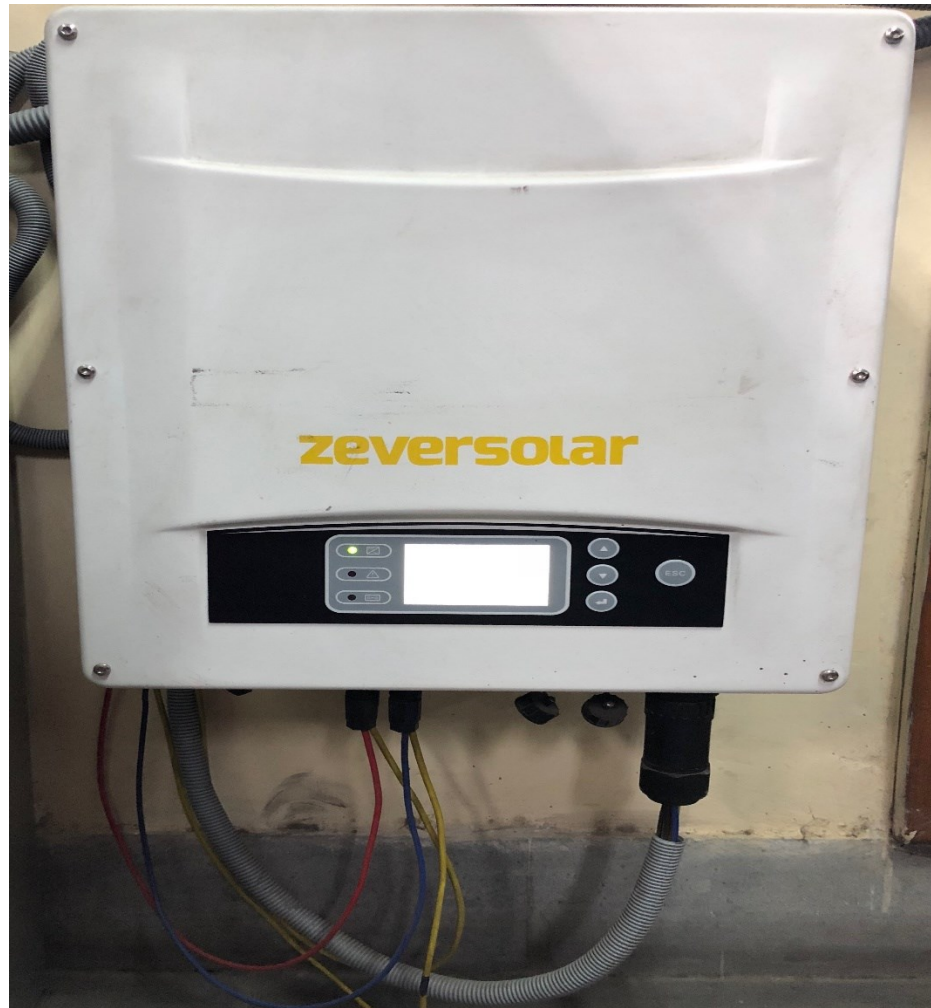
Fig. B.3 Grid connected inverter in laboratory
