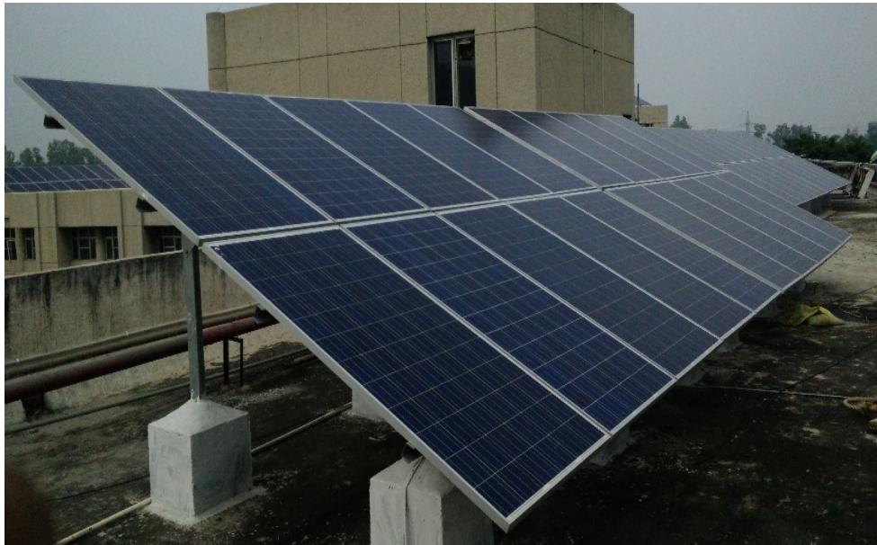
Fig. B.1 5 kW p PV system installed at roof top of EEU laboratory, DTU
