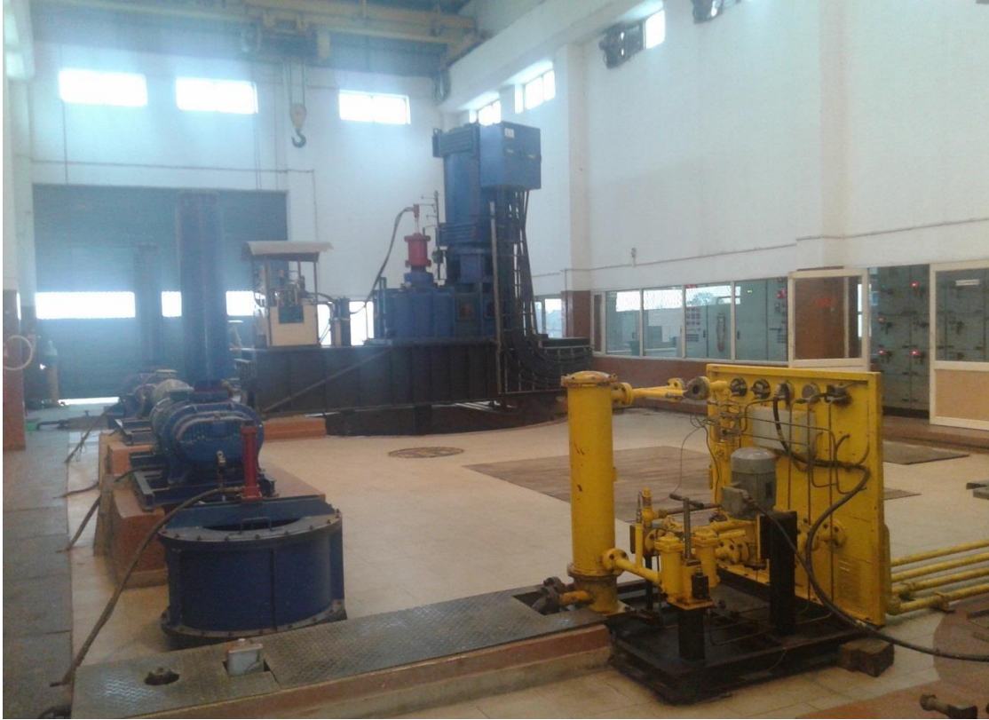
Figure 4.2: Inside View of plant
