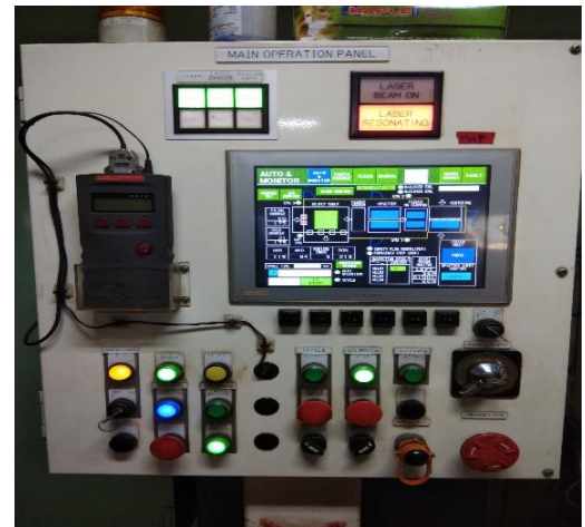
(b) Control panel
