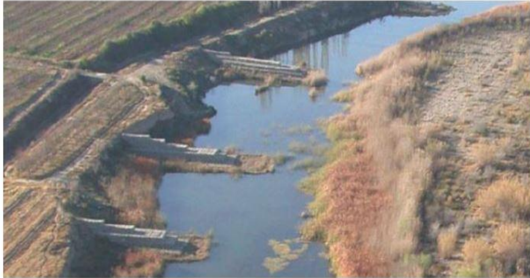
Figure.1.8 Concrete made straight groynes in a river bend on Gamka River, South Africa (Source: “The use of Groynes for Riverbank Erosion Protection”, Hans King,2009)
