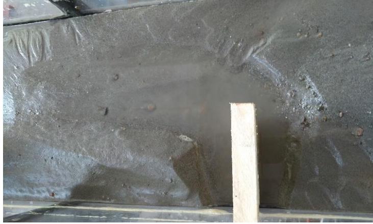
Figure 5.5.2: Scouring around second full length impermeable Groyne.
