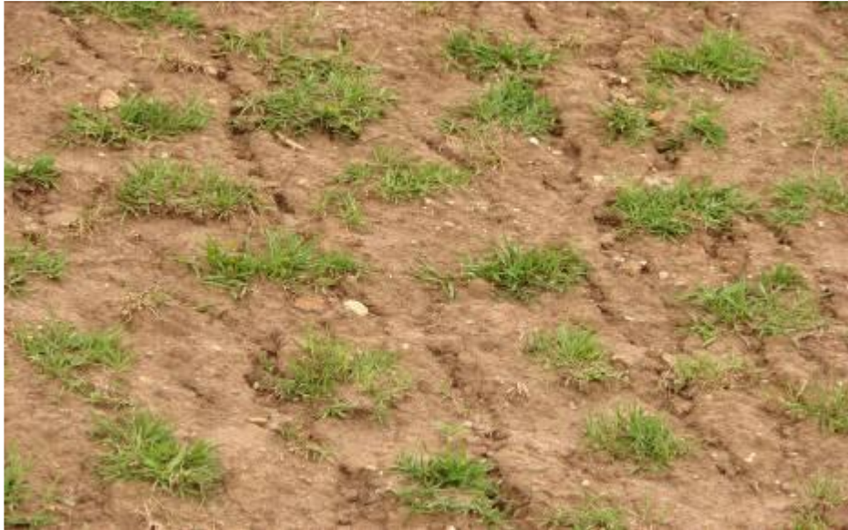
Fig 1.2: Erosion of soil of downstream face.
