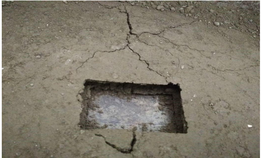
Figure 3.7 Settlement of footing
